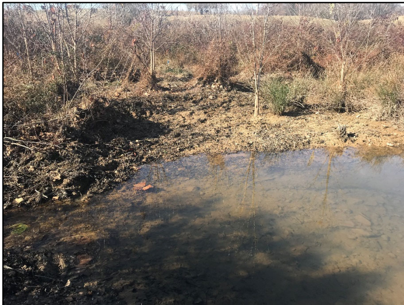
SPA 5-1 - Station 35+50 – Former beaver dam downstream of culvert caused water to back up and banks to lose vegetation (11/24/20)
