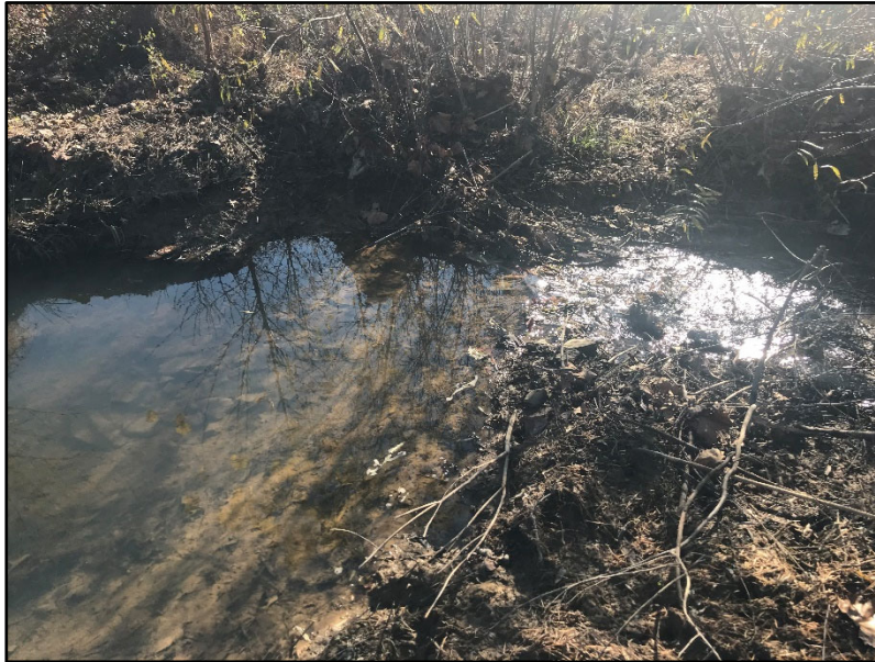
SPA 5-1 - Station 35+50 – Former beaver dam downstream of culvert caused water to back up and banks to lose vegetation (11/24/20)
