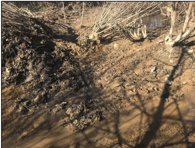
SPA 5-3 - Station 39+50 to 40+20 – Former beaver dam caused water to back up and banks to lose vegetation (11/24/20)
