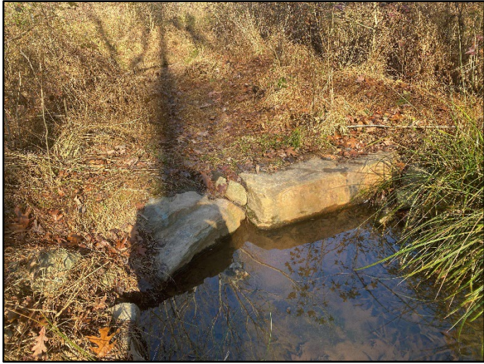
Piping Structure #1 - Unrepaired (12/3/2023)
