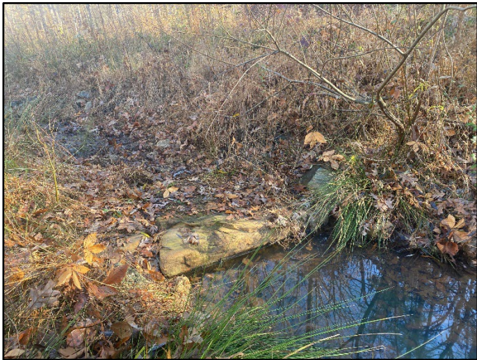
Piping Structure #3 - Unrepaired (12/3/2023)
