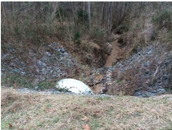
View downstream from the second crossing showing channel incision in the downstream reach of UTWB. 1/20/16
