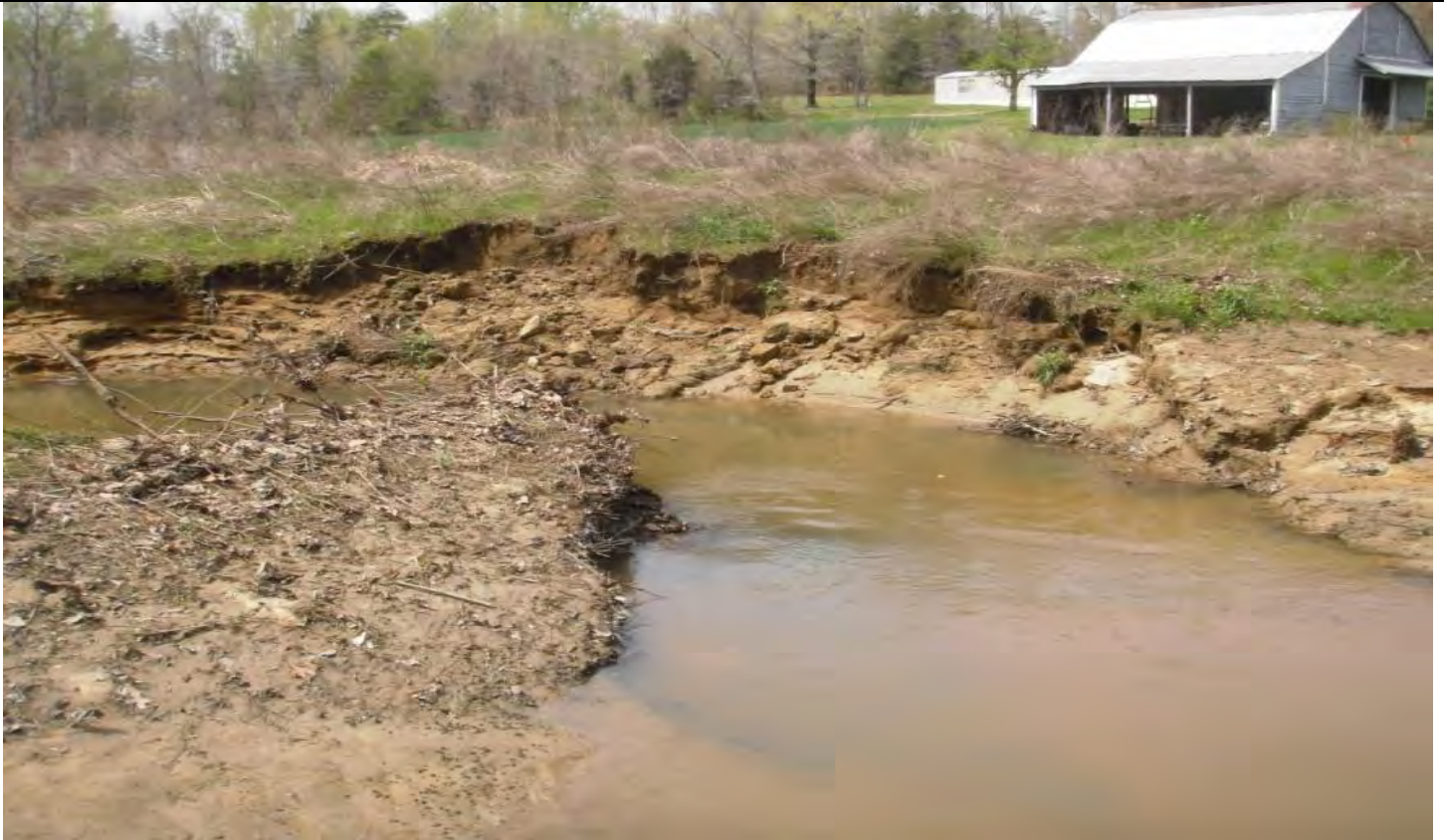
SP04 (2011) - Bank scour on right bank of Reach Lower A (STA 95+50)
