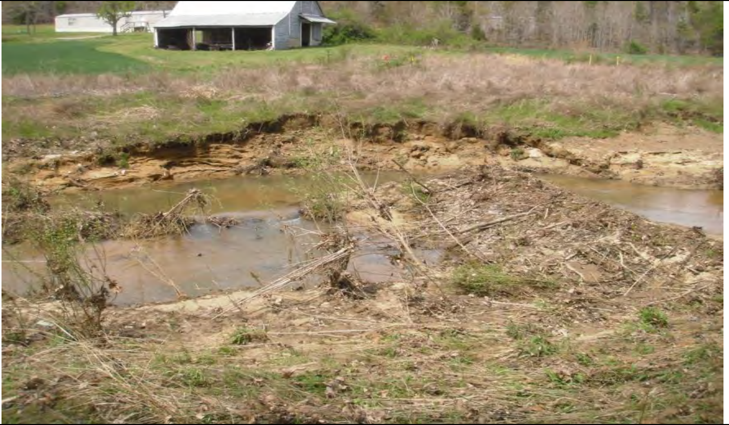
SP06 (2011) - 2-foot tall beaver dam on Reach A (STA 95+50)
