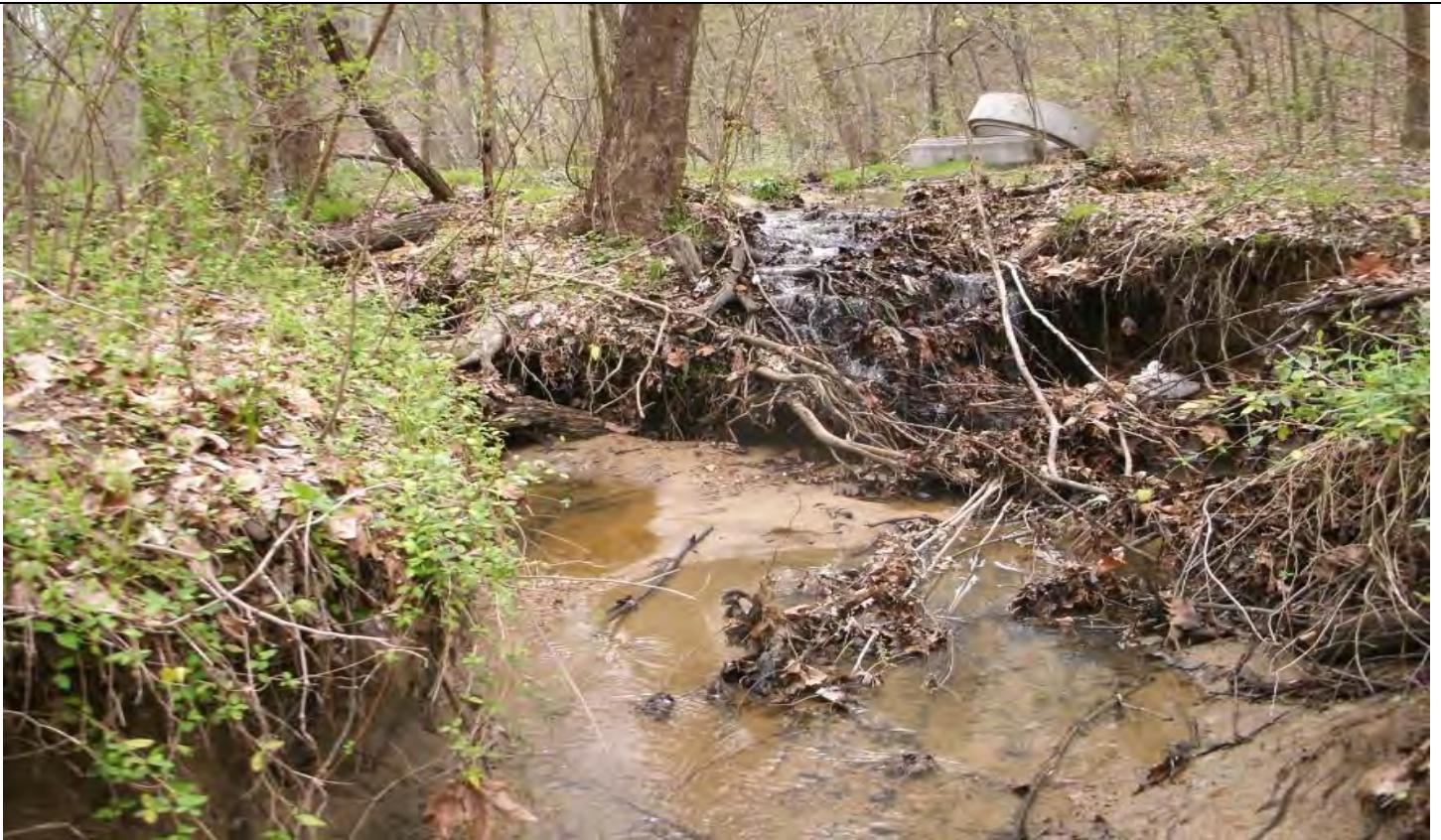
SP01 (2011) - Manhole with missing cover on Reach C (STA 100+000)
