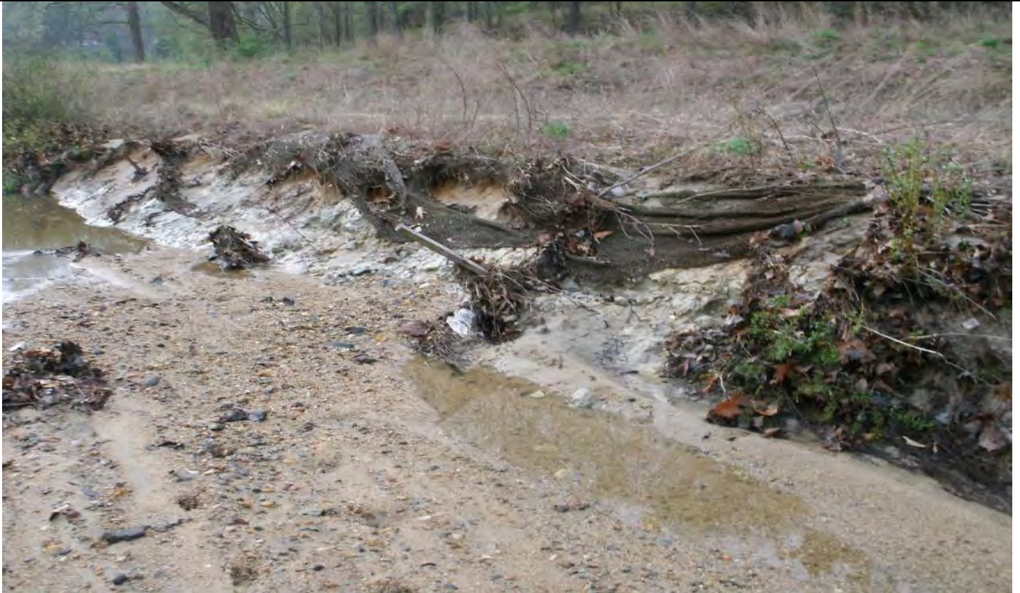
SP02 (2011) - Bank Slump on left bank of Reach B (STA 150+350)
