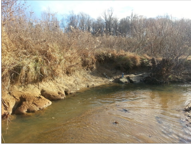
Bank erosion (Station 79+00) – 12/18/2013
