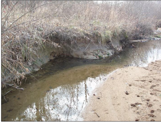
Bank erosion (Station 55+00) – 12/18/2014
