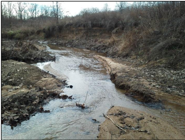
Bank erosion (Station 95+75) – 12/18/2014
