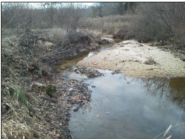
Bank erosion (Station 1515+00) and deposition (typical along Reaches A and B) – 12/18/2014
