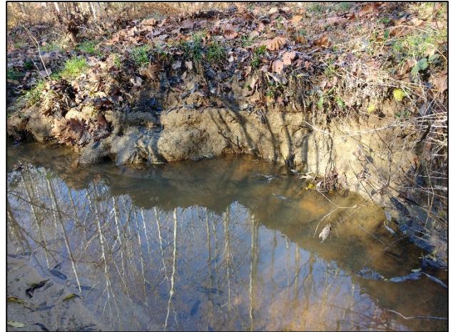
Bank erosion (Station 100+50) – 12/7/2015
