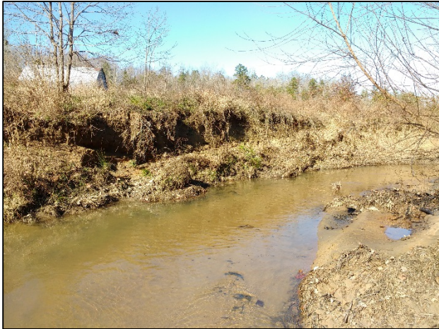
Bank erosion (Station 95+75) – 12/7/2015
