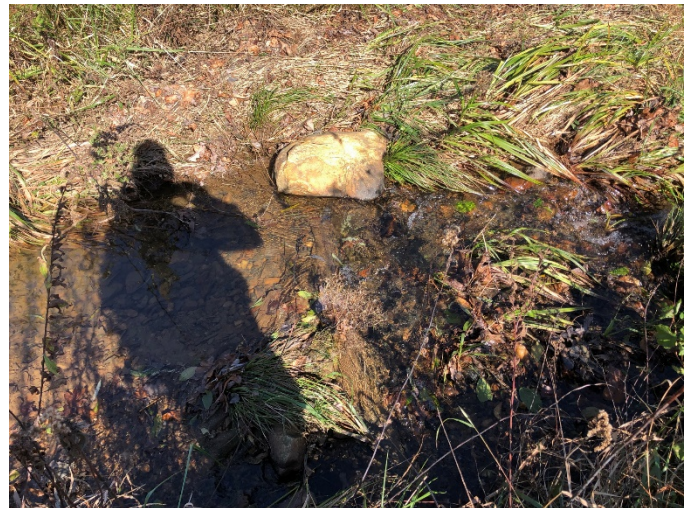
Photo 6 – UT1 R1: Station 204+90 – Structure missing. 11-6-2020
