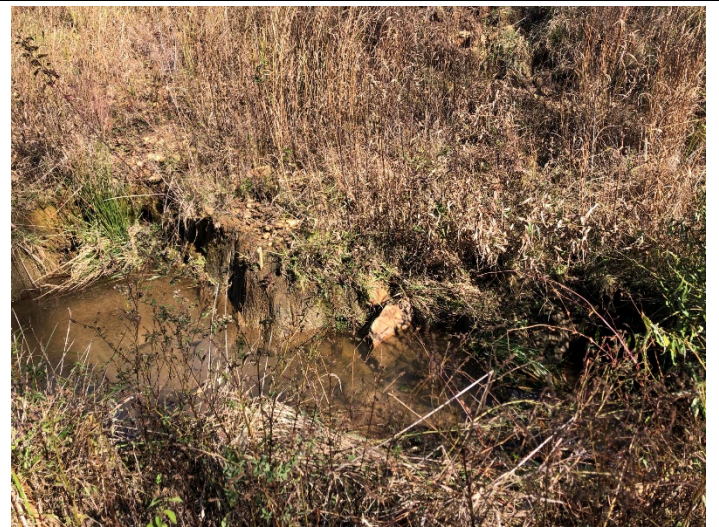
Photo 12 – UT2: Station 306+30 – 306+70 – Bank scour. 11-6-2020
