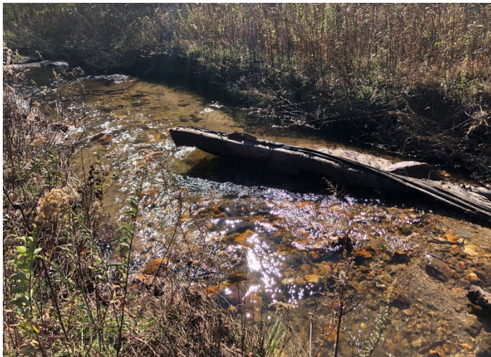
Photo 5 – Vile Creek R2: Station 122+80-123+00 – Bank scour. 11-6-2020
