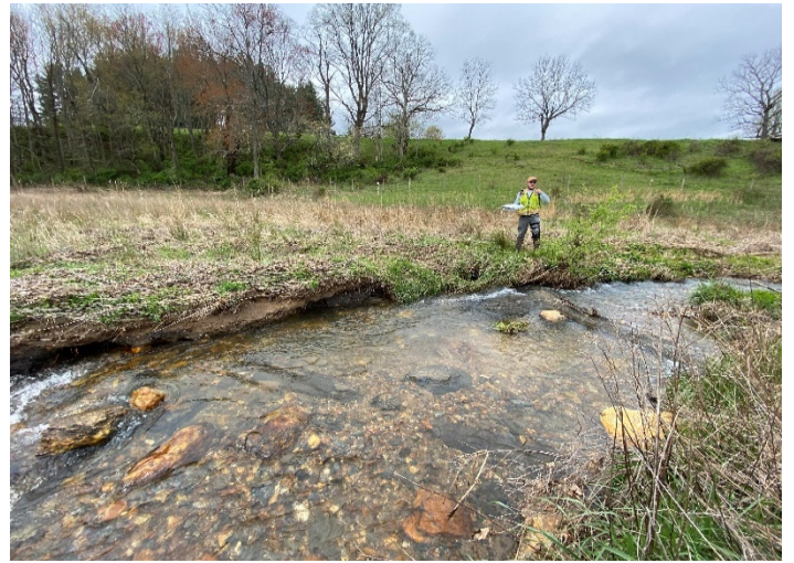
Photo 2 – Vile Creek R1: Station 103+90-104+20 – Right bank scour and piping around structures in constructed riffle. 4-14-2020
