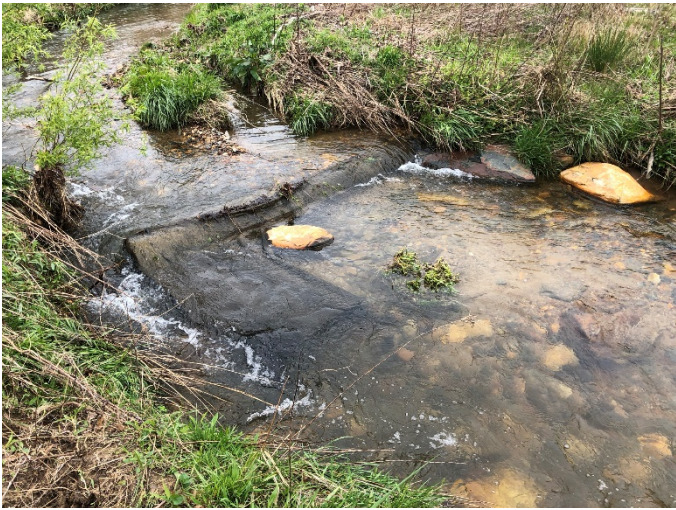
Photo 1 – Vile Creek R1: Station 103+90 – Right bank piping and scour around log sill. 4-14-2020
