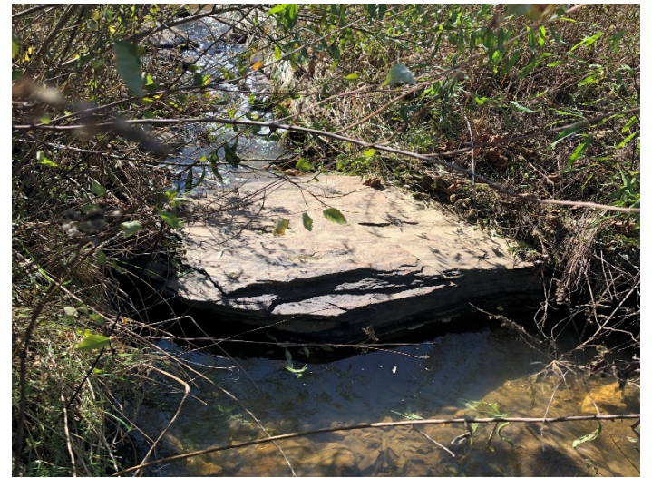
Photo 10 – UT1 R2: Station 220+98 – Piping around structure 11-6-2020
