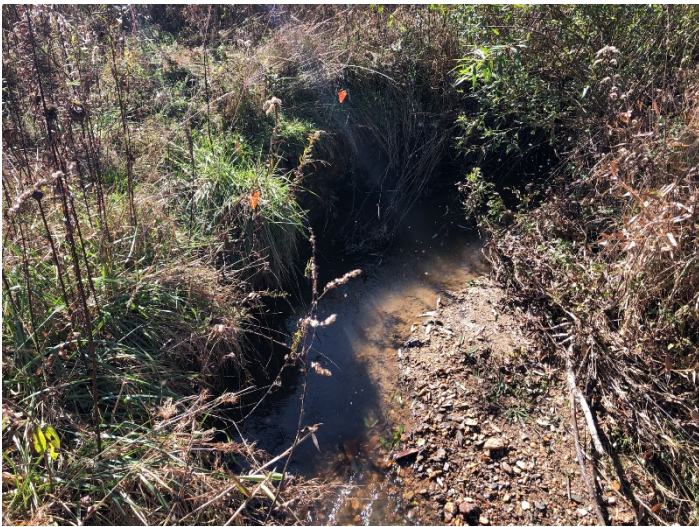
Photo 9 – UT1 R1: Station 206+40 – 206+60 – Bank Scour 11-6-2020
