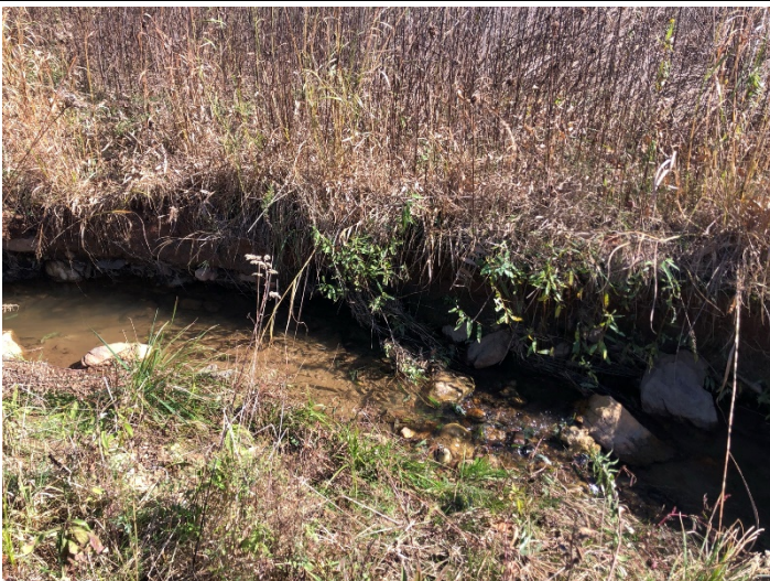
Photo 11 – UT2: Station 305+00 – 305+50 – Bank scour. 11-6-2020
