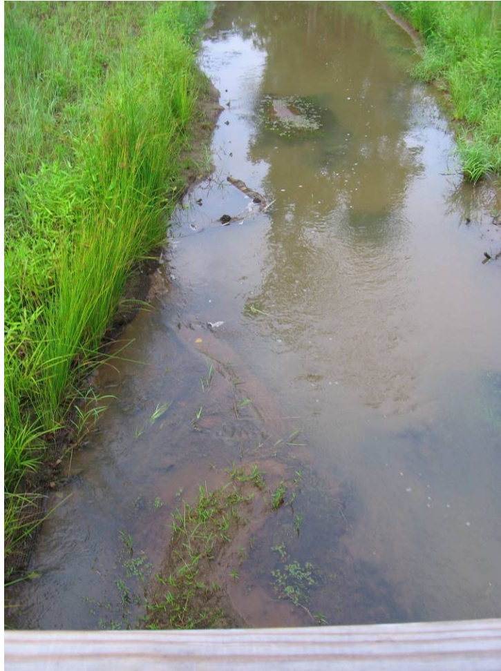
Photo 55: Problem Area III, 8+50 (0882 - Looking downstream) 06/22/05
