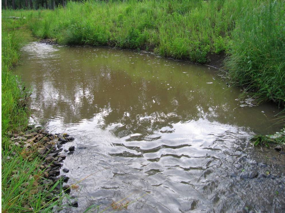
Photo 58: Problem Area VI, 15+40 (0898 - Looking upstream) 06/22/05
