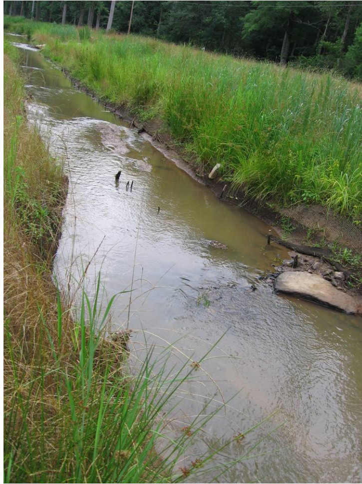
Photo 64: Problem Area X, 25+00 (0910 – Looking upstream) 06/22/05
