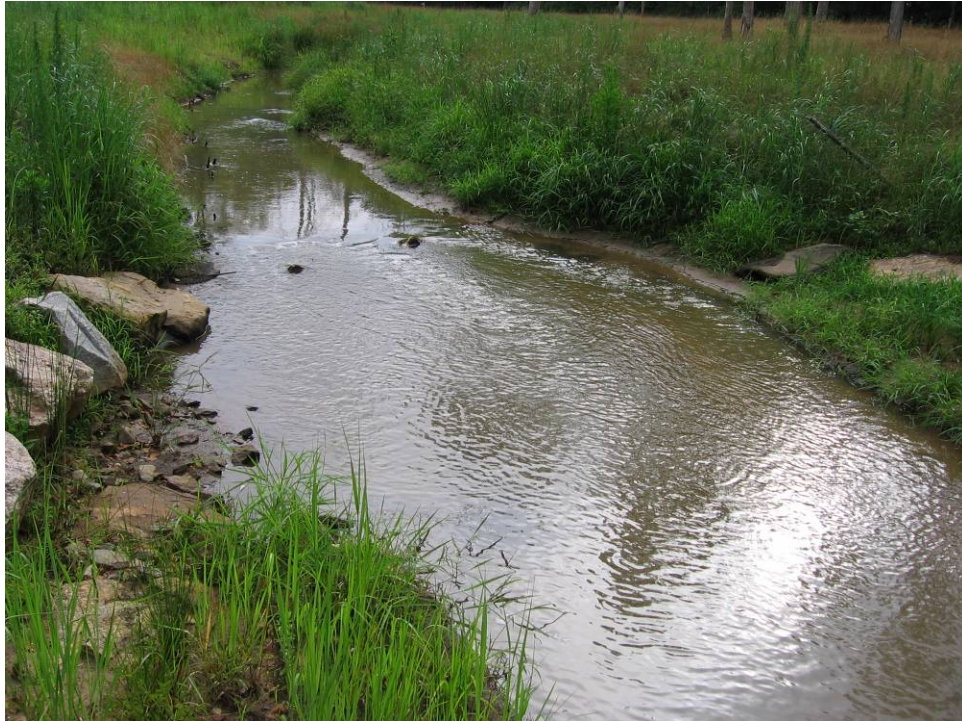
Photo 69: Problem Area XI, 26+70 (0920 – Looking upstream) 06/22/05
