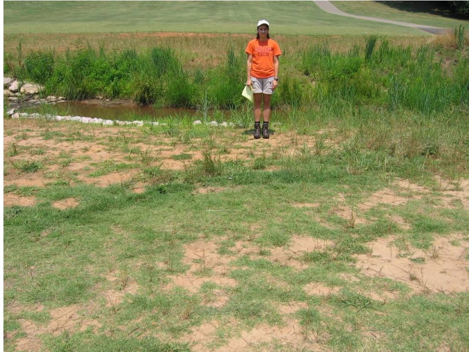
Photo 6: Vegetative Problem Area a, 0+80 – 1+40 (0780 – Left Bank) 06/22/05
