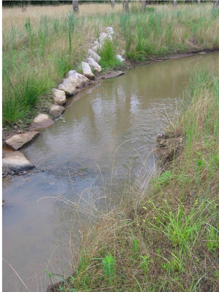
Photo 65: Problem Area X, 25+00 (0912 – Looking downstream) 06/22/05
