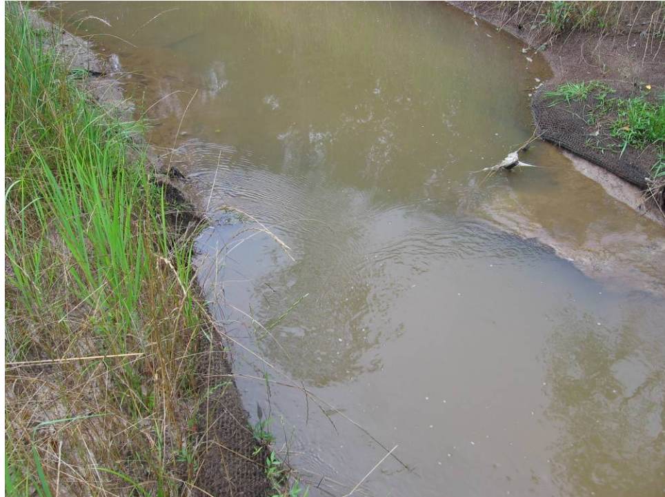
Photo 67: Problem Area X, 25+00 (0918 – From Right Bank) 06/22/05
