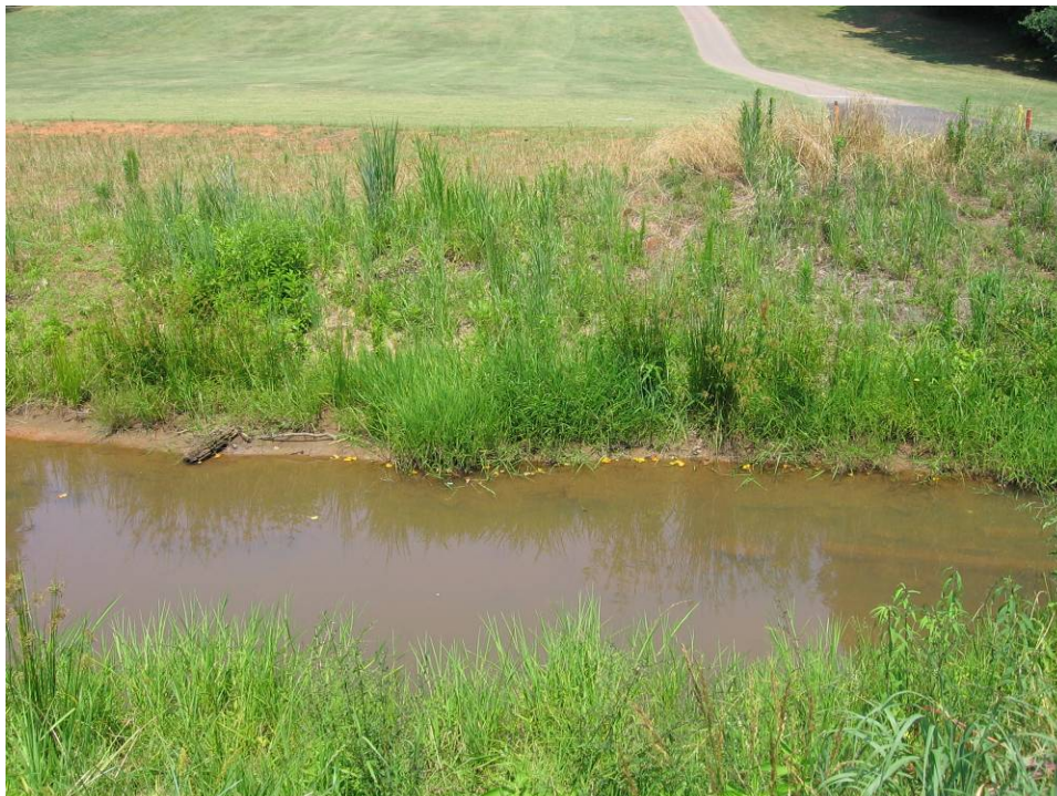
Photo 7: Vegetative Problem Area b, 0+80 – 1+40 (0783 – Right Bank) 06/22/05
