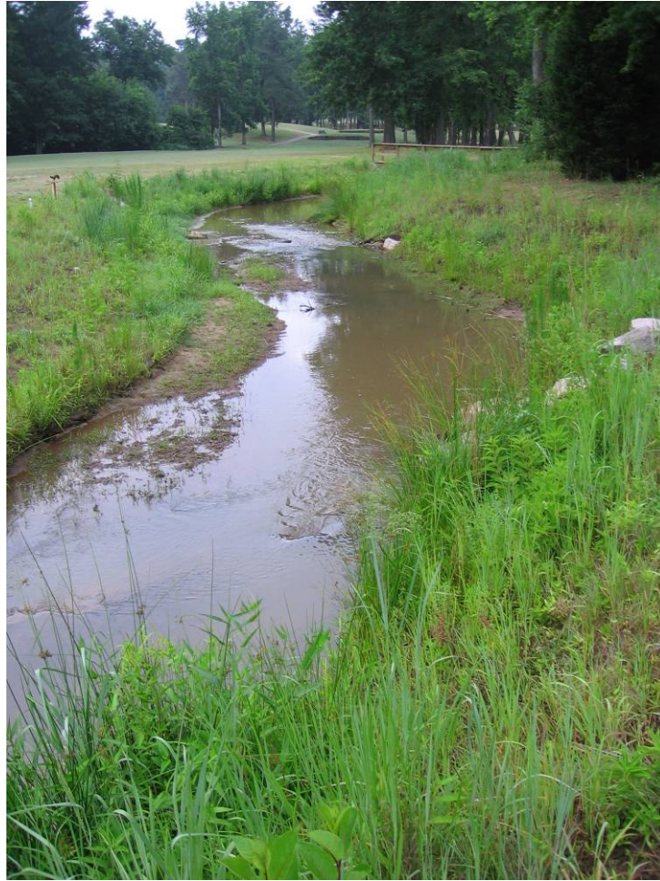
Photo 54: Problem Area II, 7+50 (0873 - Looking downstream) 06/22/05
