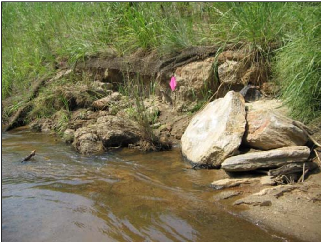
Photograph SPA-3: Engineered Structure - Back or Arm Scour, 2+85, 8.01.06
