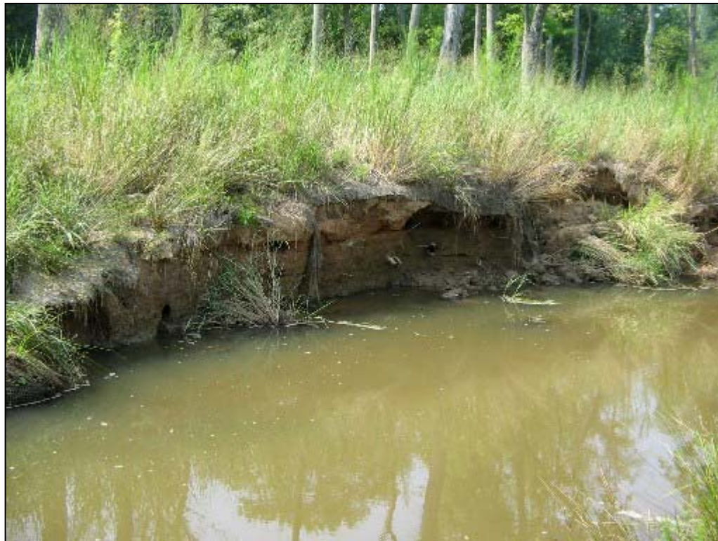
Photograph SPA-2: Bank Scour, 25+10, 8.01.06
