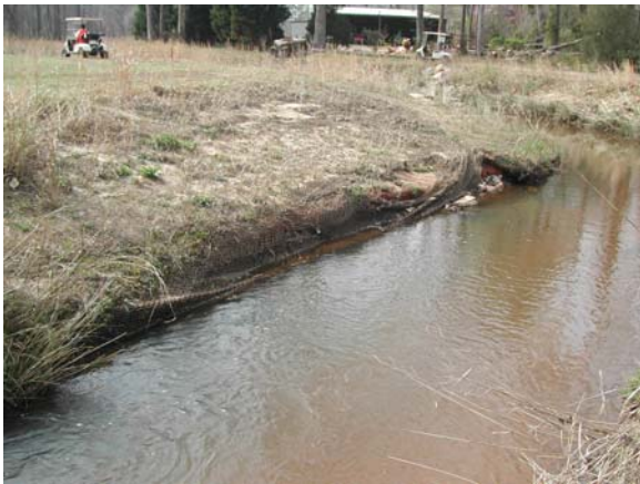
Photo 3: Representative bank erosion problem area (16+16 along mainstem).
