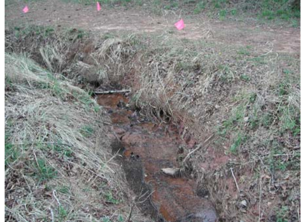
Photo 2: Representative undercut problem area (11+43 along unnamed tributary) at left toe (photo facing upstream).
