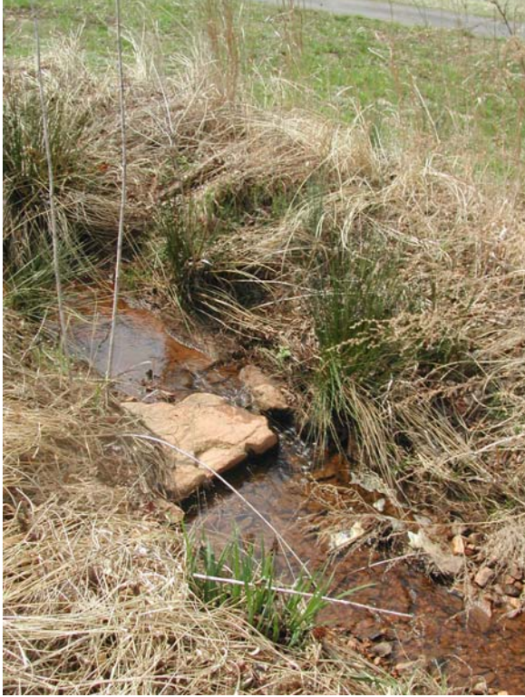
Photo 5: Representative problem crossvane (13+99 along unnamed tributary).
