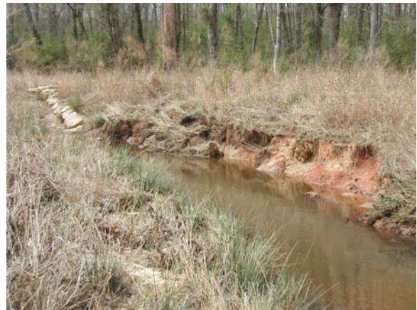
Photo 4: Representative severe bank erosion problem area on the right bank (37+86 along mainstem).
