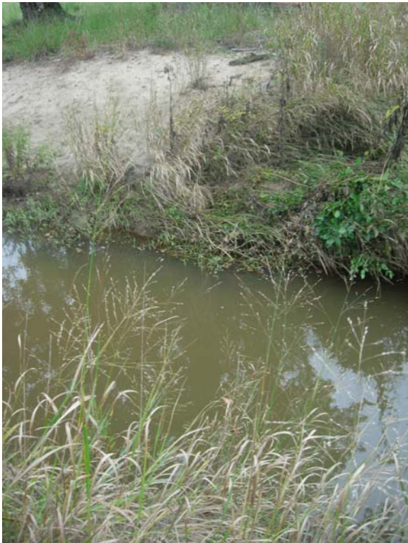
Photo 3. Representative bare bench/bank problem area (Station 16+56; view of left bank on main stem; 9-30-2008).
