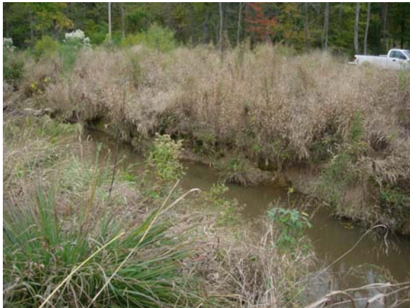
Photo 3: Representative severe bank erosion problem area (Station 34+28; view upstream of left bank along Horse Creek; 10-29-2008).
