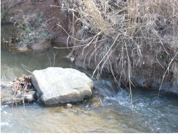
Photo 5: Representative j-hook problem area, Horse Creek (Station 37+07 view upstream of piping along left side of structure; 2-15-2008).
