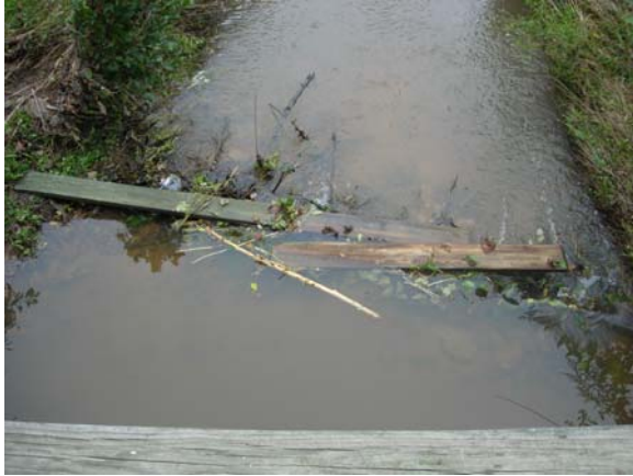
Photo 1: Representative beaver-dam problem area (Station 10+98; view downstream along Horse Creek; 9-30-2008).
