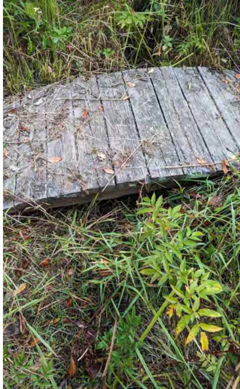
Permanent Photo Point 20: Footbridge crossing on UT 8 upstream end, facing downstream (Taken 9/27/23)
