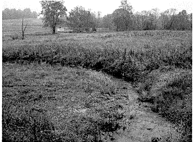
Photograph 42. Looking downstream from culvert at log vane, log toe protection, and root wads installed between LT Stations 10+87 and 11+85. (9/27/04)
