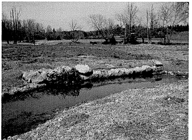
Photograph 36. Looking downstream at root wad and log toe protection installed between LT Stations 10+10 and 10+30. (4/7/04)
