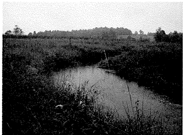
Photograph 64. Looking downstream at log toe protection and root wads installed between MS Stations 30+80 and 30+00. (9/27/04)
