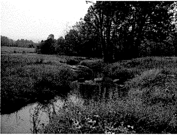
Photograph 127. Looking upstream from MS Station 2+90 at log J vane installed at MS Station 3+53. (9/27/04)
