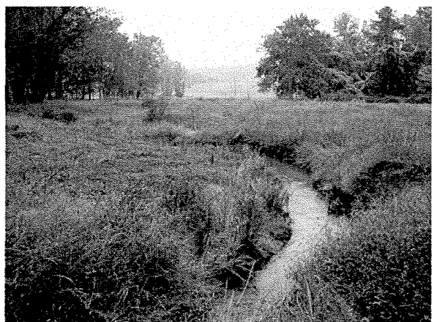
Photograph 12. Looking downstream at log vane, root wad, and log toe protection installed between LT Stations 2+65 and 3+20. (9/27/04)
