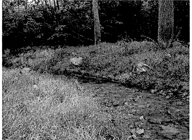
Photograph 4. Looking downstream at log toe protection installed between LT Stations 1+50 and 1+90 to protect large trees. (9/27/04)
