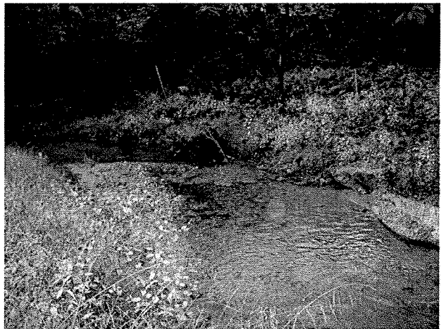
Photograph 6. Looking downstream from rock J vane at root wads and log vane installed between MC Stations 2+20 and 2+57. (9/27/04)
