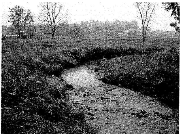
Photograph 48. Looking downstream at log vane, root wads, and log toe protection installed between MC Stations 19+97 and 20+75. (9/27/04)
