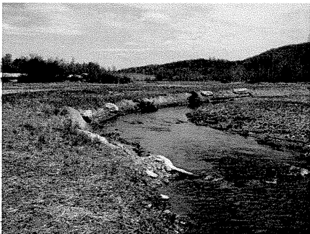
Photograph 37. Looking downstream at rock cross vane installed at MS Station 44+38 and root wads/log toe protection. (4/7/04)
