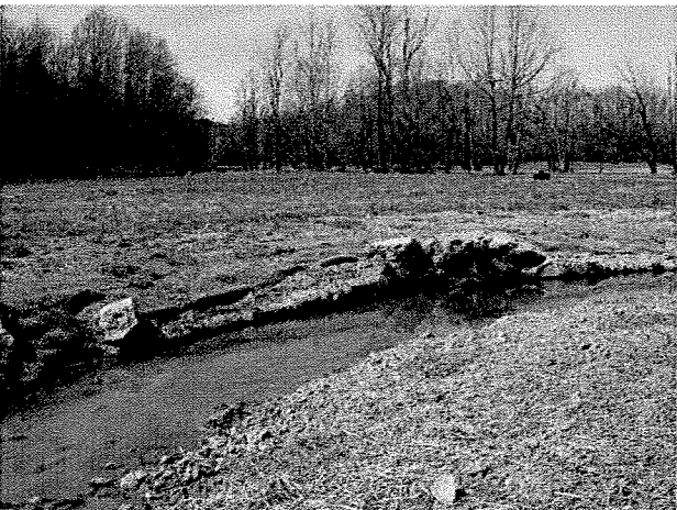
Photograph 35. Looking downstream at log toe protection and root wad installed between LT Stations 10+60 and 10+80. (4/7/04)
