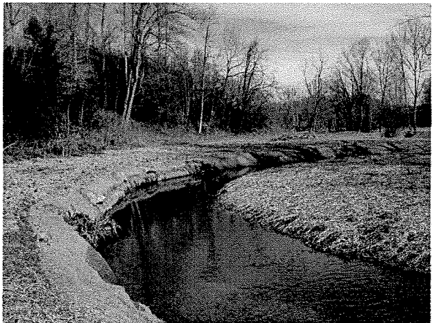
Photograph 18. Looking downstream at root wads and log toe protection installed between MC Stations 8+70 and 9+40. (1/16/04)
