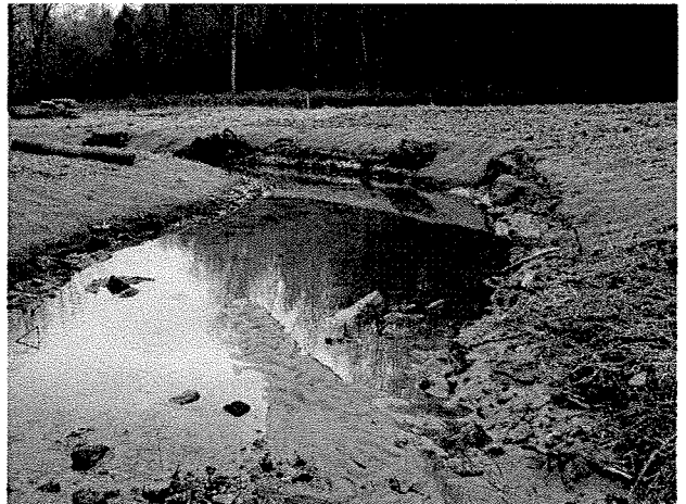
Photograph 12. Looking downstream at rock J vane installed at MC Station 5+86 and log toe protection and root wads installed between MC Stations 6+20 and 6+55. (12/18/03)
