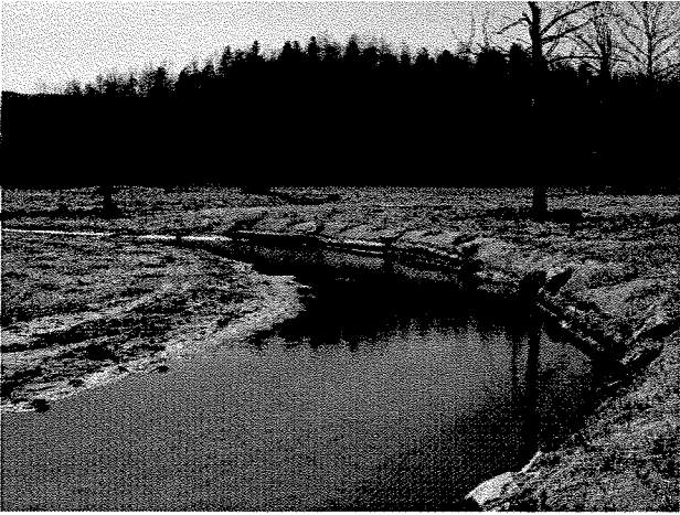
Photograph 103. Looking upstream at log toe protection and root wads installed between MS Stations 12+65 and 11+15. (4/7/04)
