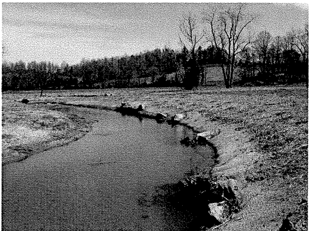
Photograph 90. Looking downstream at log toe protection and root wads installed between MS Stations 18+00 and 17+00. (4/7/04)
