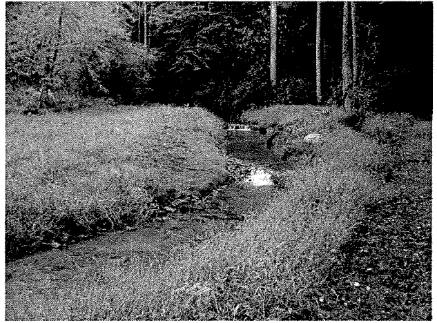
Photograph 2. Looking upstream at rock cross vane, log toe protection, root wads, and log vane installed between MC Stations 0+12 and 1+08. (9/27/04)
