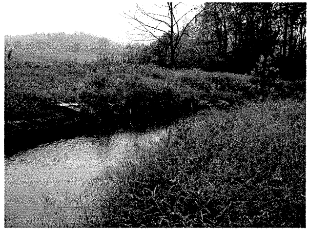
Photograph 122. Looking upstream at root wads and log toe protection installed between MS Stations 4+35 and 3+90. (9/27/04)
