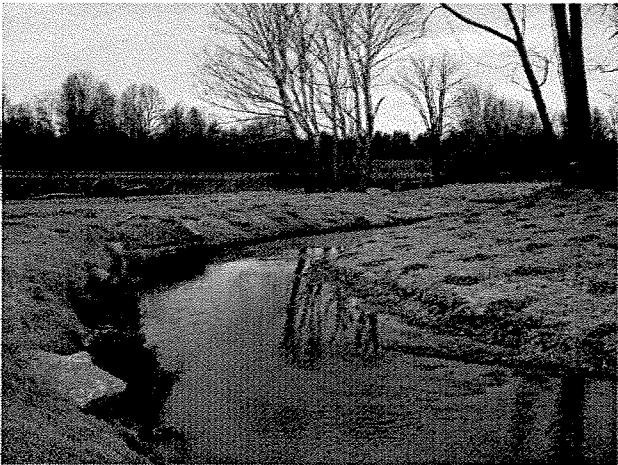
Photograph 117. Looking downstream at root wads and log toe protection installed between MS Stations 6+10 and 5+40. (4/7/04)
