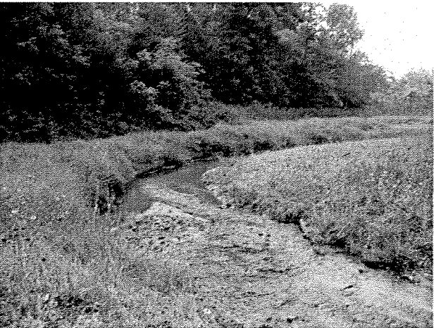
Photograph 17. Looking downstream at rock cross vane installed at MC Station 8+25 and root wads and log toe protection installed between MC Stations 8+70 and 9+20. (9/27/04)
