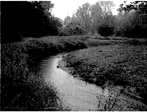
Photograph 19. Looking downstream at root wads and log toe protection installed between MC Stations 8+70 and 9+40. (9/27/04)
