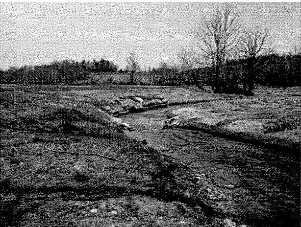
Photograph 71. Looking downstream at rock cross vane, log toe protection, and root wad installed between MS Stations 27+33 and 26+25. (4/7/04)
