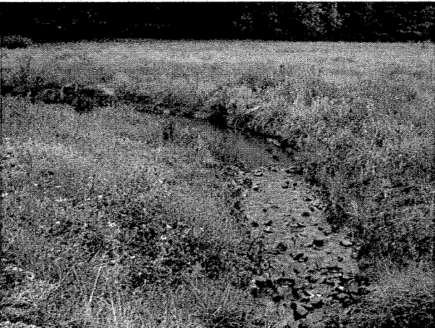
Photograph 41. Looking upstream from culvert at log toe protection and root wads installed between LT Stations 9+65 and 10+30. (9/27/04)
