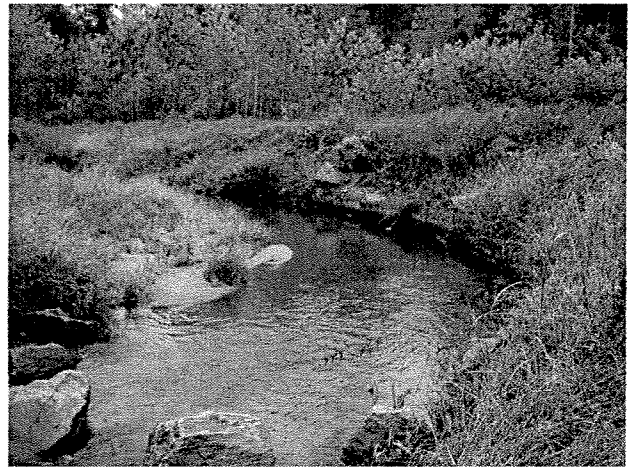
Photograph 26. Looking downstream at rock J vane installed at MS Station 53+01 and downstream log toe protection/root wad. (9/27/04)
