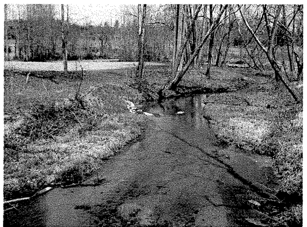
Photograph 4. Looking downstream from culvert at rock J vane installed in existing MS channel. (4/7/04)
