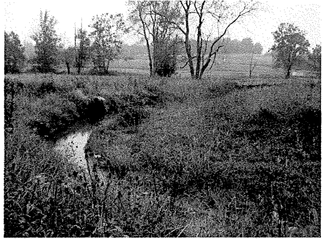
Photograph 38. Looking downstream at log vane, root wads, and log toe protection installed between LT Stations 9+44 and 10+30. (9/27/04)
