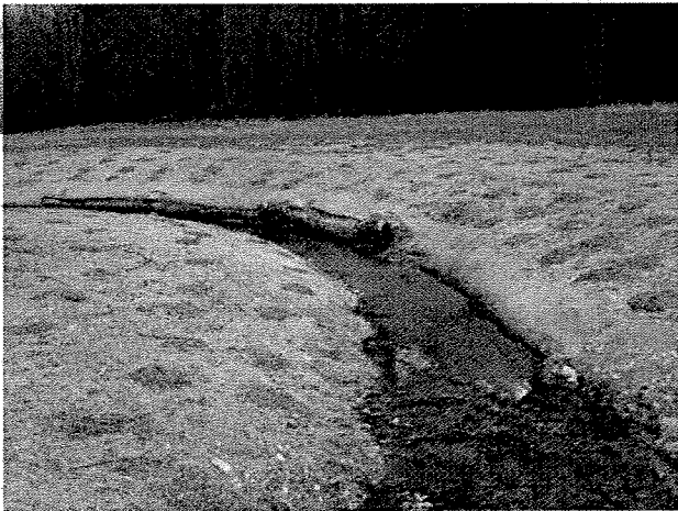
Photograph 33. Looking downstream from culvert at log vane, root wads, and log toe protection installed between MC Stations 13+66 and 15+85. (4/7/04)
