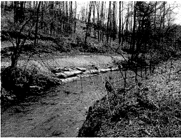
Photograph 1. Looking upstream from culvert at log toe protection installed on banks of existing MS channel at upstream end of project area. (4/7/04)
