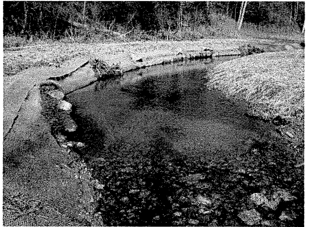
Photograph 16. Looking downstream at rock cross vane installed at MC Station 8+25 and root wads and log toe protection installed between MC Stations 8+70 and 9+20. (1/16/04)
