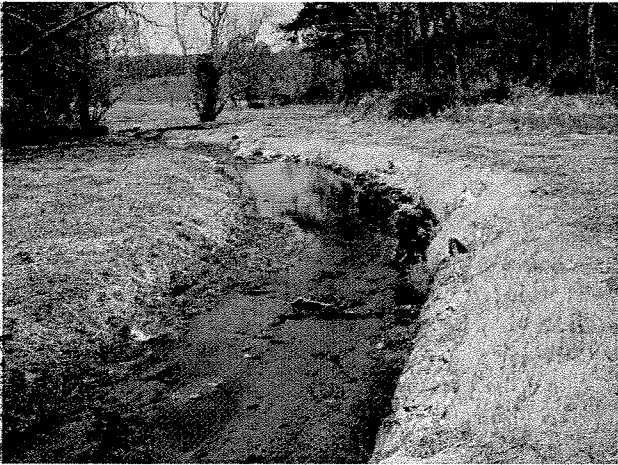
Photograph 3. Looking downstream at log toe protection and root wads installed between LT Stations 0+25 and 0+95. (4/7/04)
