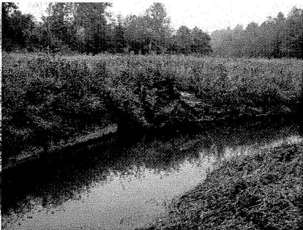
Photograph 99. Looking upstream from left bank at log toe protection and root wads installed between MS Stations 14+15 to 13+70. (9/27/04)
