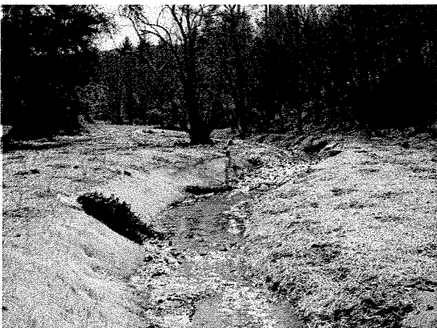
Photograph 11. Looking upstream at log vane and root wad installed between LT Stations 2+65 and 2+90. (4/7/04)
