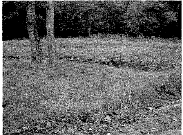
Photograph 34. Looking across culvert at root wads and log toe protection installed on right bank between MC Stations 14+00 and 14+70. (9/27/04)
