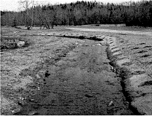
Photograph 61. Looking downstream at rock J vane, log toe protection, and root wads installed between MS Stations 32+50 and 31+50. (4/7/04)
