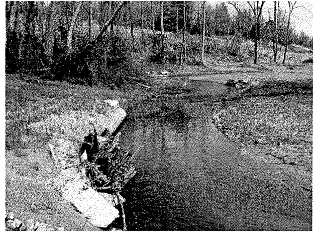
Photograph 14. Looking downstream from MS Station 60+50 at root wad and log toe protection. (4/7/04)
