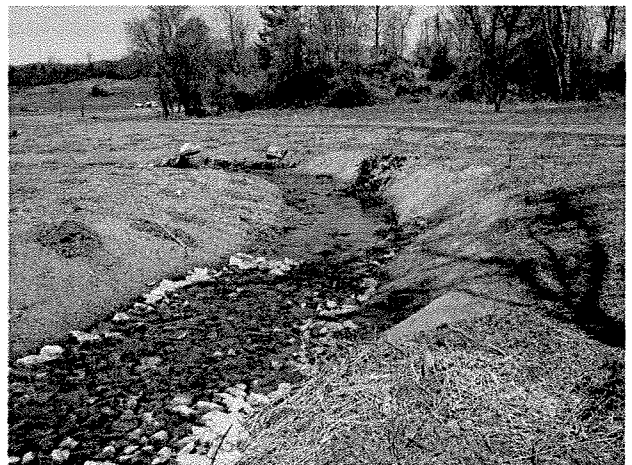
Photograph 10. Looking downstream at log vane, root wad, and log toe protection installed between LT Stations 2+65 and 3+20. (4/7/04)
