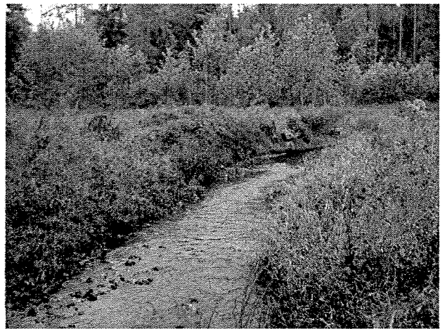
Photograph 28. Looking upstream at log toe protection and log vane installed at MS Station 51+93. (9/27/04)
