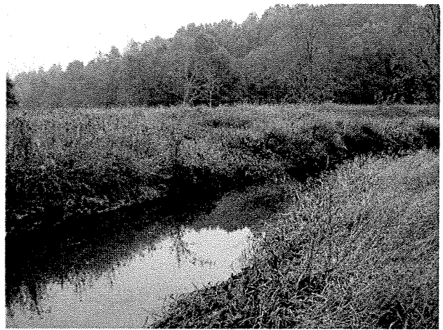
Photograph 98. Looking upstream from left bank at log toe protection and root wads installed between MS Stations 14+25 to 13+90. (9/27/04)
