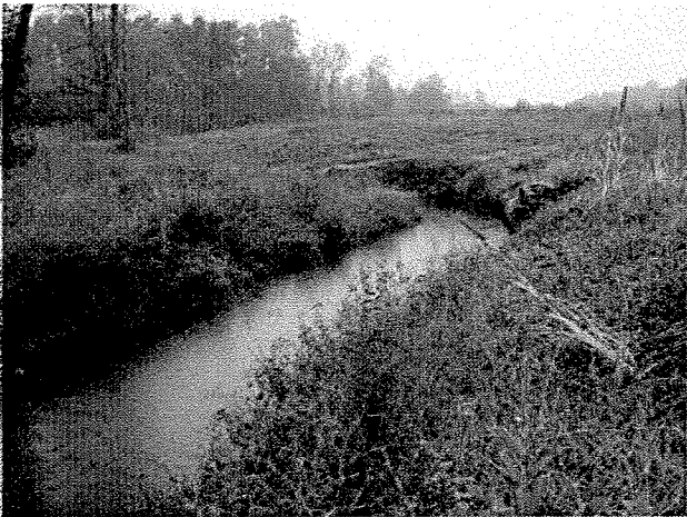
Photograph 81. Looking upstream at root wad and log toe protection installed between MS Stations 20+90 and 20+60. (9/27/04)
