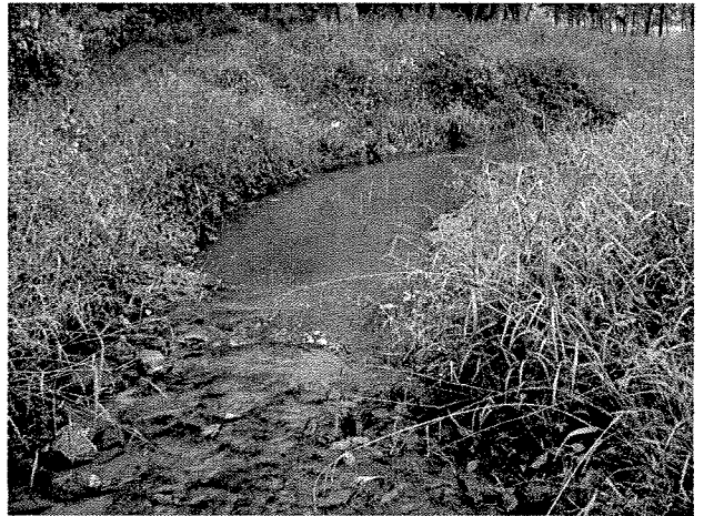
Photograph 16. Looking downstream at rock cross vane and root wad installed between LT Stations 3+58 and 3+90. (9/27/04)
