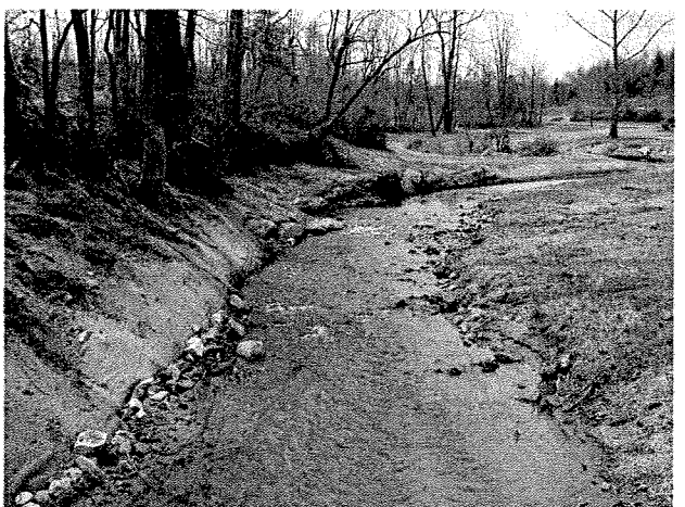
Photograph 54. Looking upstream at rock toe protection, root wads, and rock vane installed between MS Stations 34+75 and 33+75. (4/7/04)
