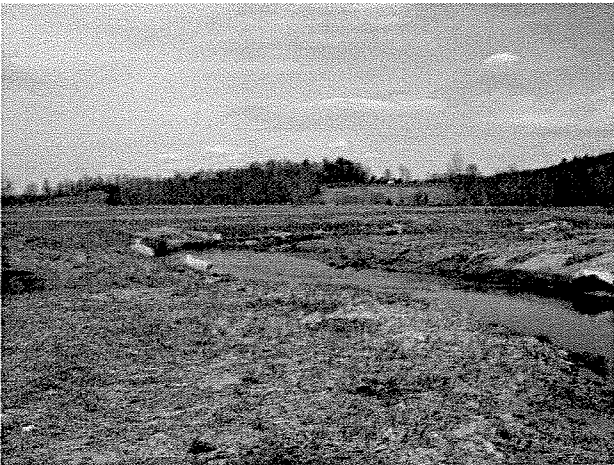
Photograph 63. Looking downstream at log toe protection and root wads installed between MS Stations 30+80 and 30+00. (4/7/04)
