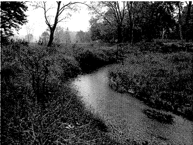
Photograph 29. Looking downstream from LT Station 12+10 at root wads installed between MC Stations 12+45 and 12+65. (9/27/04)
