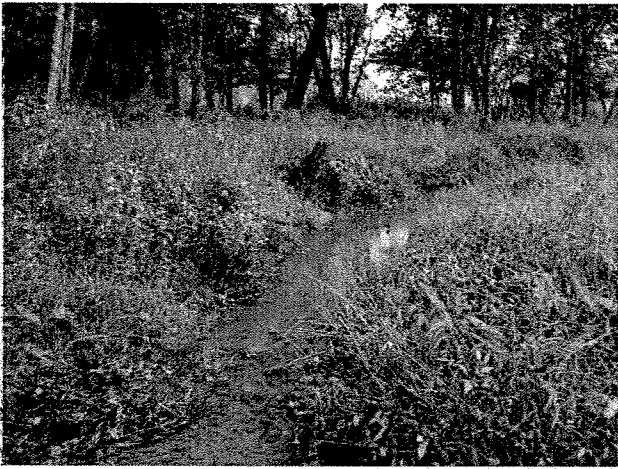
Photograph 25. Looking downstream at root wad and log toe protection installed between LT Stations 6+25 and 6+60. (9/27/04)
