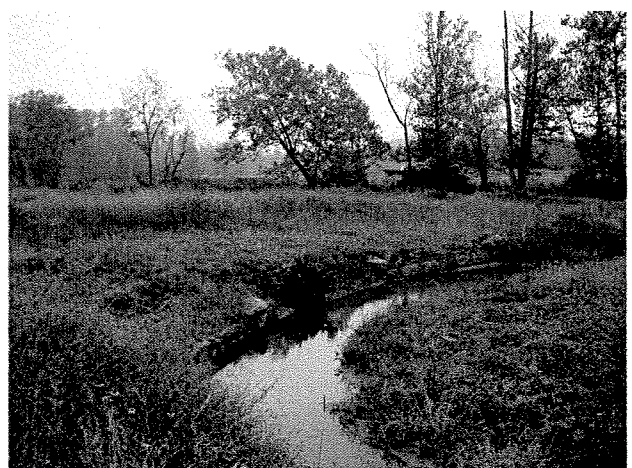
Photograph 46. Looking downstream at log toe protection, root wad, and log vane installed between LT Stations 12+60 and 13+23. (9/27/04)
