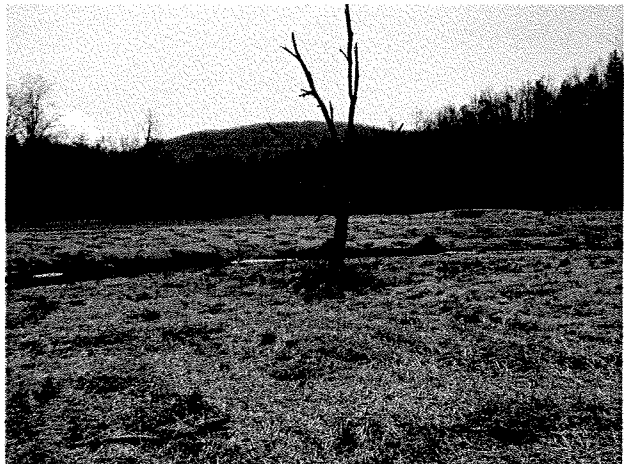
Photograph 96. Log toe protection and root wads installed around bend between MS Stations 14+55 and 13+90 (preserved snag on left bank). (4/7/04)
