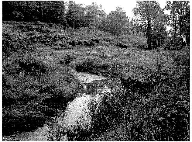
Photograph 22. Looking downstream at root wads and log vane installed at MS Station 55+08. (9/27/04)
