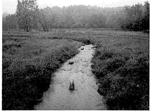
Photograph 62. Looking downstream at rock J vane, log toe protection, and root wads installed between MS Stations 32+50 and 31+50. (9/27/04)
