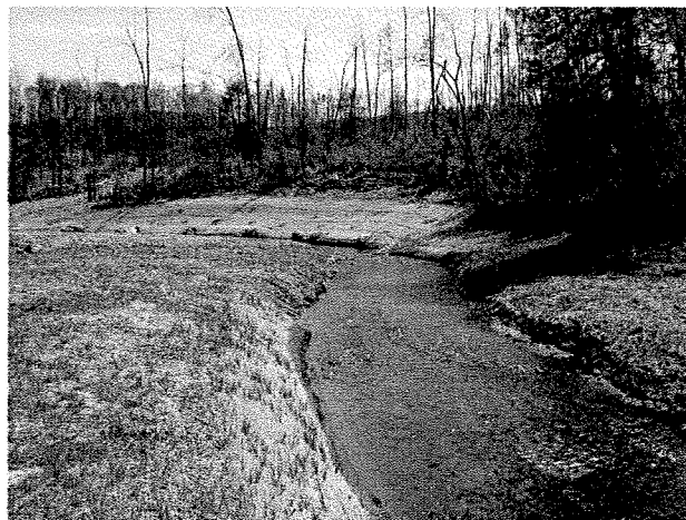
Photograph 38. Looking downstream from MS Station 43+00 at rock vane installed at MS Station 42+32 and log toe protection/root wads. (4/7/04)
