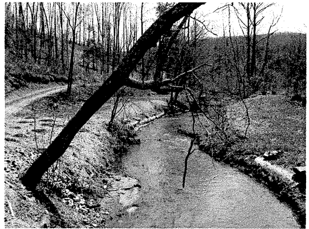
Photograph 2. Looking upstream from culvert at log toe protection installed on banks of existing MS channel at upstream end of project area. (4/7/04)
