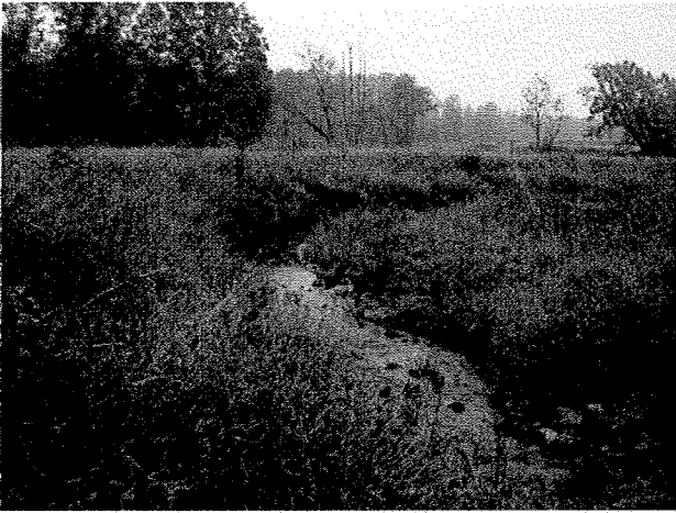
Photograph 37. Looking downstream at log vane, root wads, and log toe protection installed between LT Stations 9+44 and 10+30. (9/27/04)
