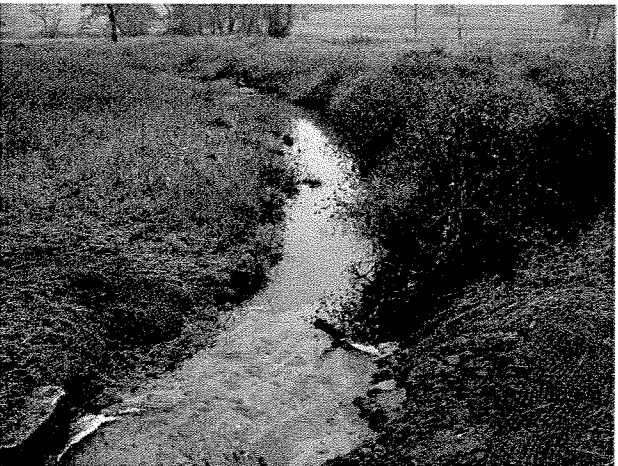
Photograph 29. Looking downstream from LT Station 7+85 at root wad and log toe protection installed between LT Stations 7+75 and 8+25. (9/27/04)
