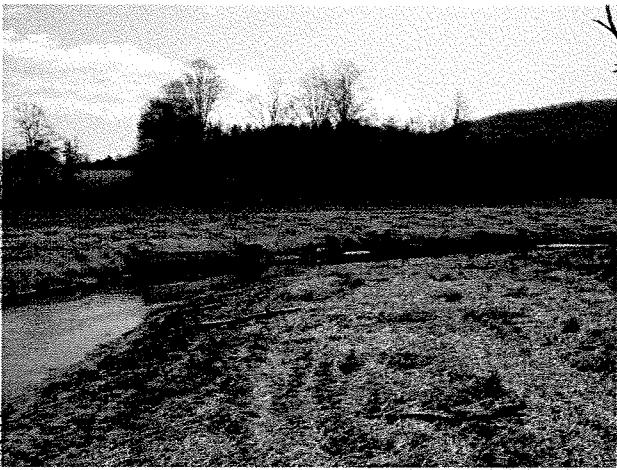
Photograph 97. Looking upstream at log toe protection and root wads installed around bend between MS Stations 14+10 and 13+45. (4/7/04)
