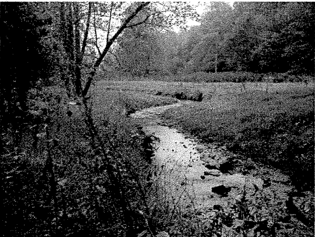
Photograph 11. Looking downstream from MC Station 4+65 at log toe protection and root wads installed on left bank between MC Stations 5+05 and 5+70. (9/27/04)
