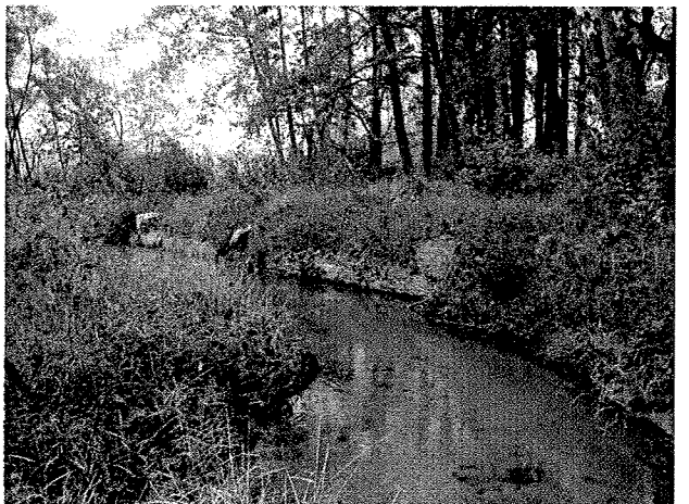
Photograph 42. Looking downstream from MC Station 17+98 at log toe protection and root wads installed between MC Stations 18+25 and 19+25. (9/27/04)
