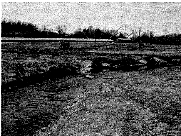
Photograph 42. Looking downstream from MS Station 40+50 at rock J vane installed at MS Station 39+98 and log toe protection/root wads. (4/7/04)
