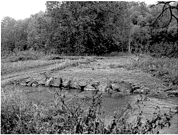
Photograph 85. Rock toe protection installed between MS Stations 19+25 and 18+80 upstream of ford crossing. (9/27/04)
