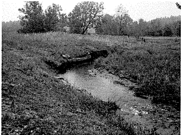
Photograph 78. Looking downstream at rock vane, root wad, and log toe protection installed between MS Stations 21+34 and 20+60. (9/27/04)
