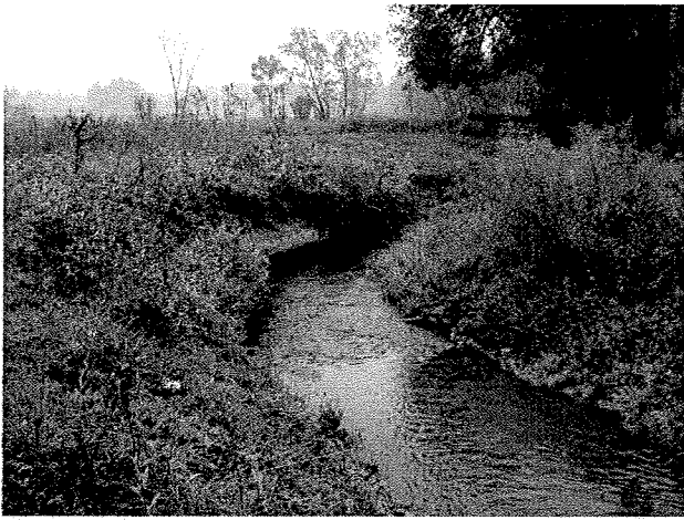
Photograph 37. Looking downstream at log vane, log toe protection, and root wad installed between MC Stations 16+03 and 16+55. (9/27/04)
