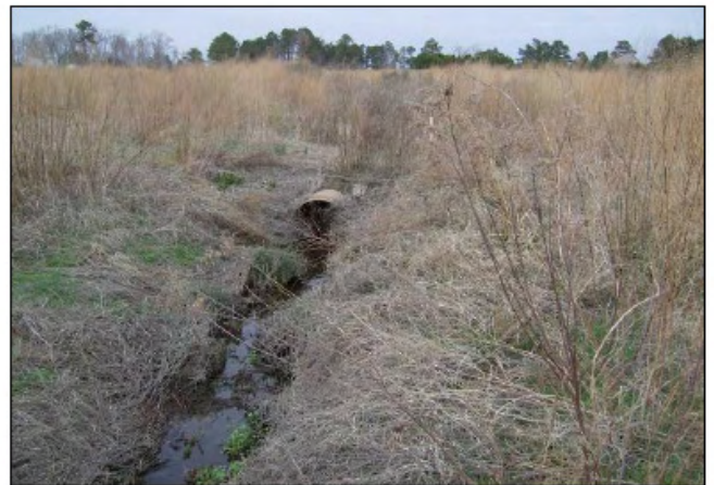
Facing northeast (upstream) at 24-inch pipe situated along middle reach of UT
