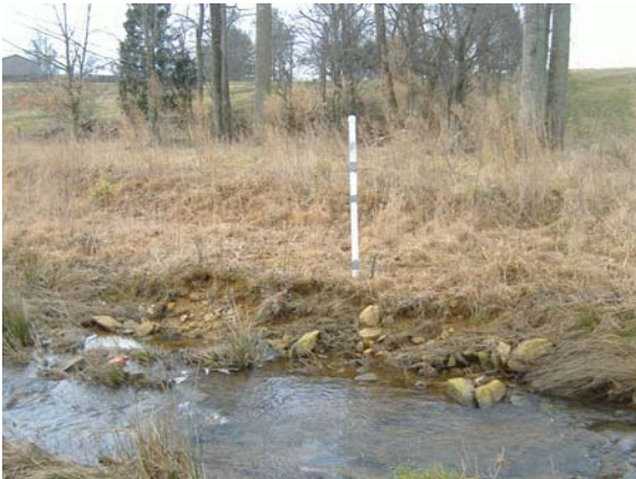
Photo 2: Bank erosion (Station 22+20 along plan view).
