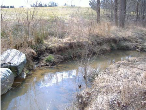
Photo 1: Bank Erosion April 11 DSCN 5750 (Station along plan view).
