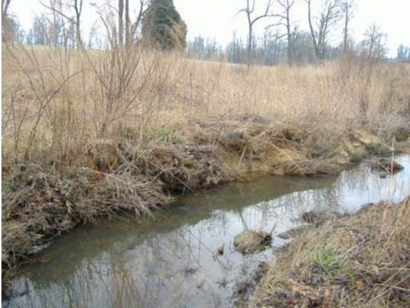
Photo 1: Bank Erosion (Station 10+85 along plan view).
