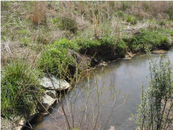
Photo2: Representative problem j-hook and bank erosion (10+10.93 along plan view).
