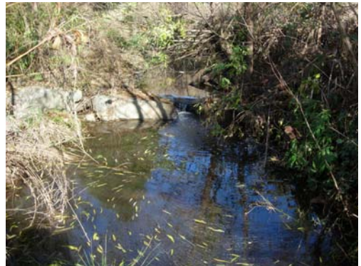
Photo 4: Representative crossvane problem area (Station No. 12+75; view upstream; 11-6-2008).
