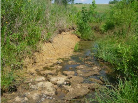
Photo 1: Representative bank erosion problem area (Station No. 17+11; view upstream; 6-17-2008).
