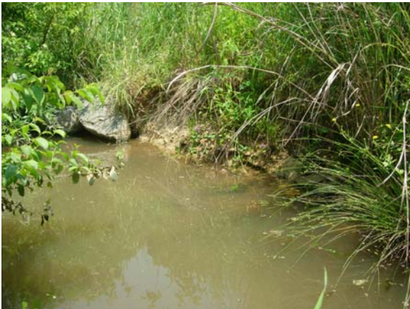
Photo 2: Representative bank erosion problem area (Station No. 10+11; view downstream of left bank; 6-10-2008).
