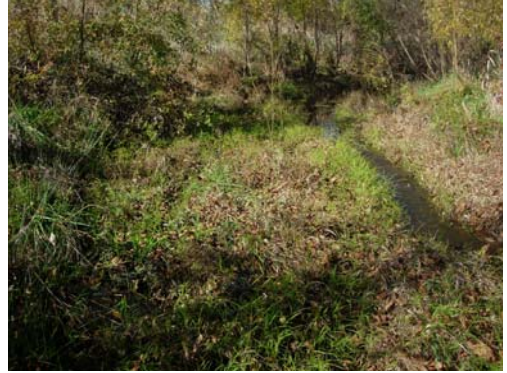
Photo 2: Representative aggradation problem area (Station No. 15+74; view downstream; 11-6-2008).
