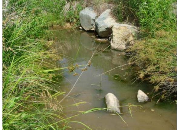
Photo 2: Representative problem j-hook and bank erosion (Station No. 17+74; view downstream; 6-17-2008).
