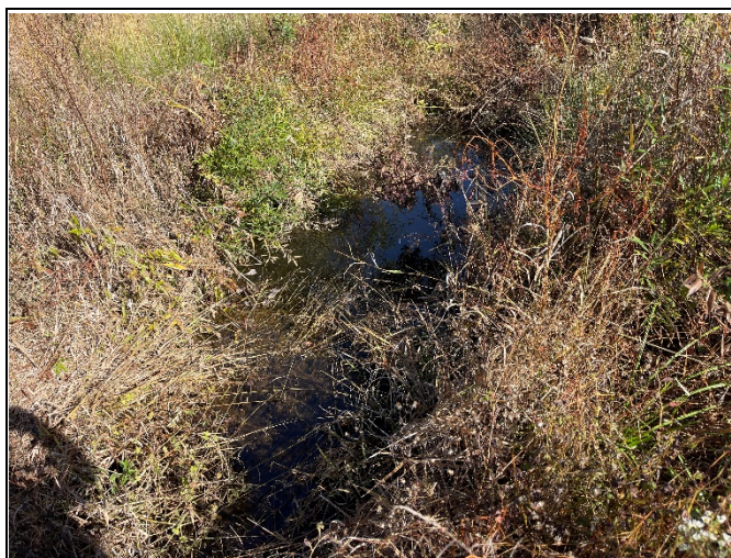
PP-27: Reach UT4B, upstream, Station 18+00
