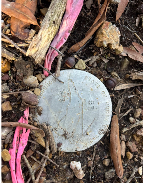
Missing caps and unmarked caps addressed, taken December 21, 2023
