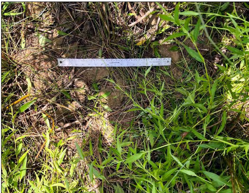
Photo 5: Soil cracking – mid-Summer conditions
