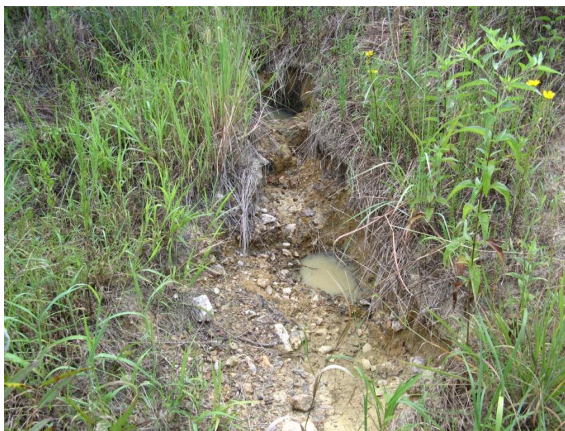
Photo 3.1.3-1 – Eroding swale through buffer
