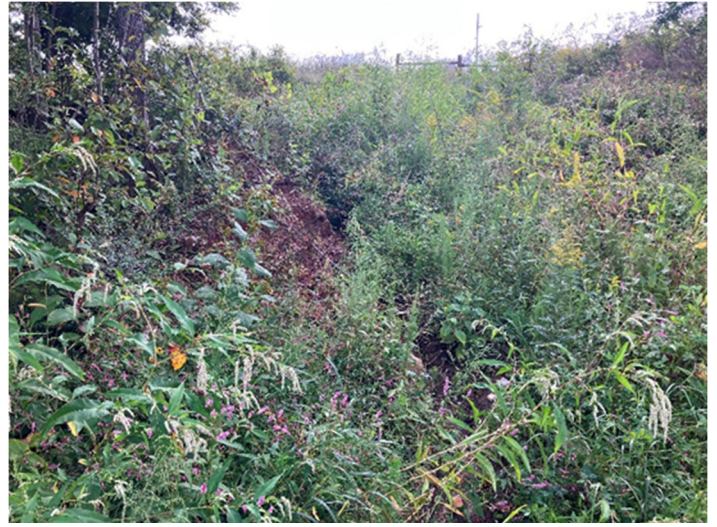
UT2 R1 – Erosion Gully next to BMP 3 (10/3/2022)
