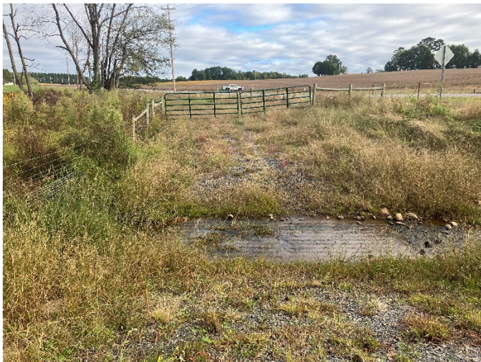
Wyant Road Ford – Improved Erosion Mitigation (10/3/2022)
