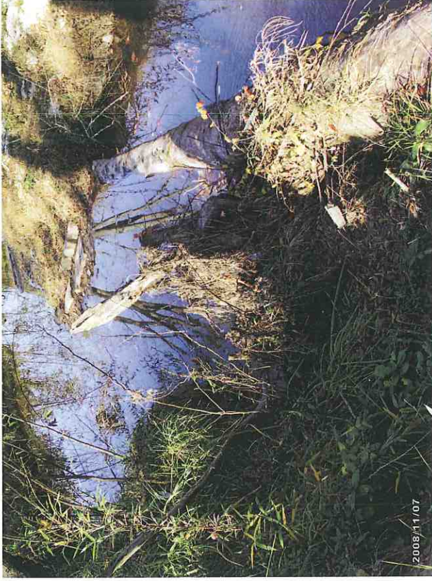
Problem Area 6 - log vane beginning to backcut
