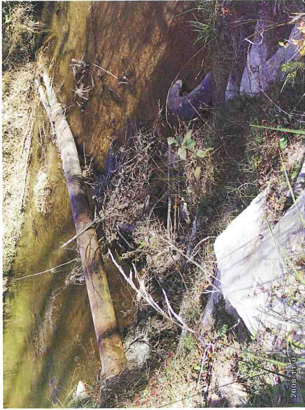
Problem Area 5 - pipe and debris, partial occlusion
