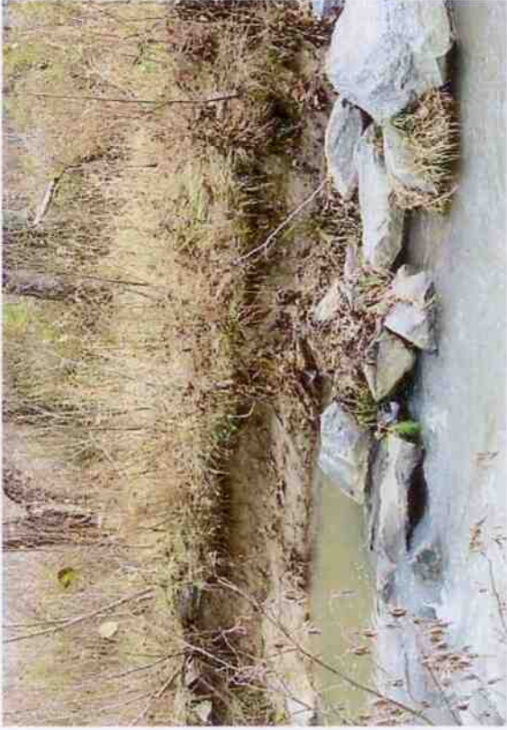
Problem Area 1 - Left Bank Scour
