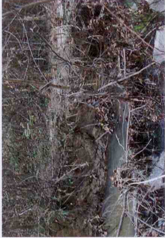
Problem Area 3 - Left Bank Scour
