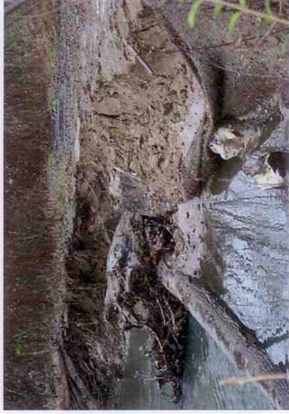
Problem Area 4 - Log vane displacement
