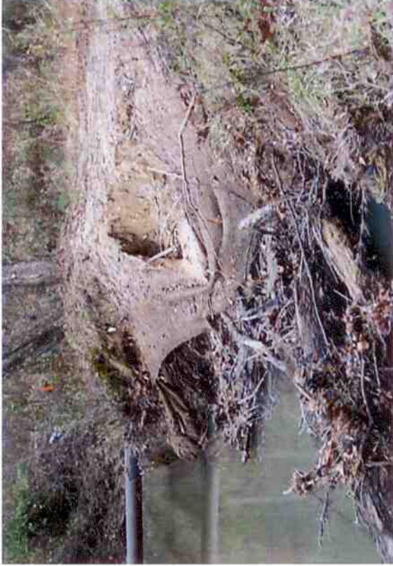
Problem Area 5 - Right Bank Failure
