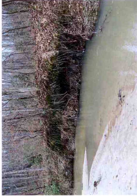
Problem Area 7 - Left Bank Scour
