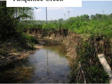
Bank erosion on Town Creek
