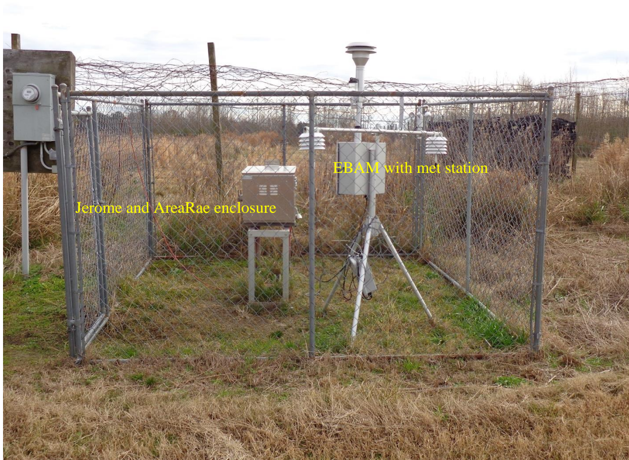
Figure 3 Williamsdale Farm Site – Typical Site Installation
