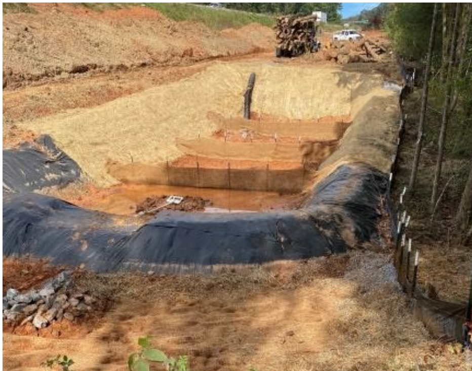
Photo-Recently Installed Basin (10/14/21)
