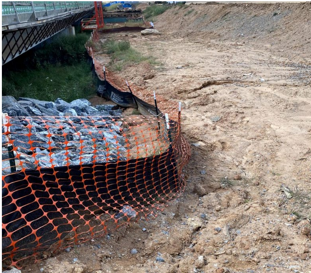
Photo- Safety Fence draped on the upstream side of silt fence (9/29/21)
