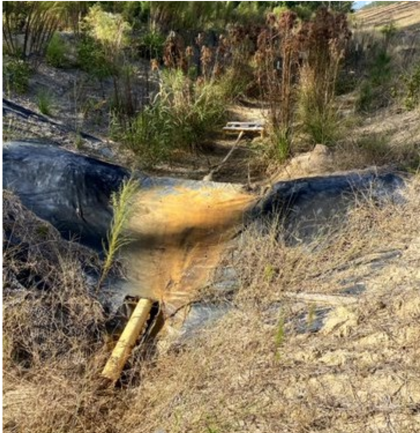
Photo- Earthen Dam with Skimmer (10/4/21)
