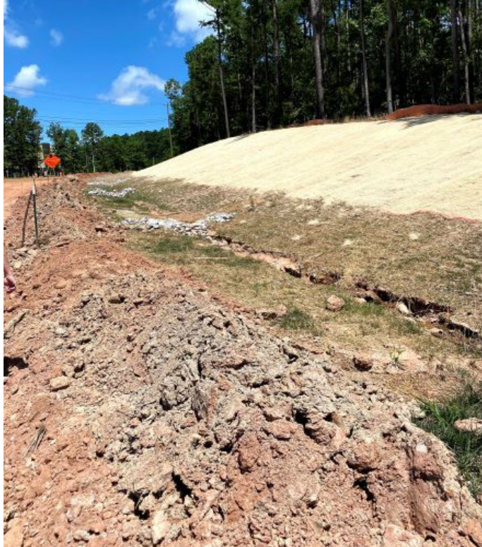
Photo- Ditch bottom beginning to erode. (7/14/2021)
