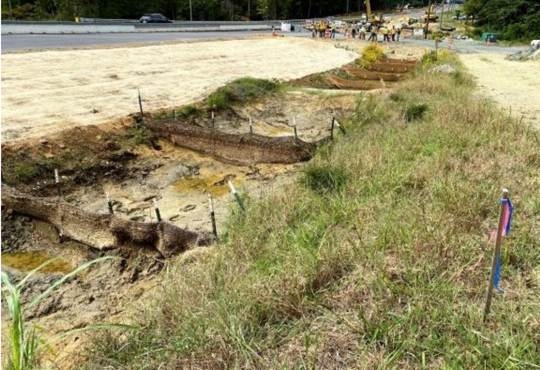
Photo- Tiered Skimmer Basin (9/17/21)
