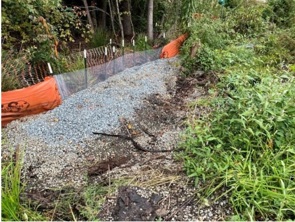
Photo- Special Sediment Control Fence adjacent to Wetlands (9/17/21)
