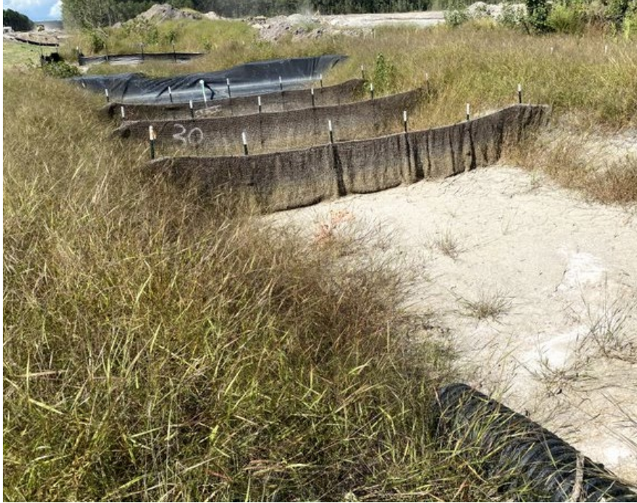
Photo- Skimmer Basin. (10/4/21)
