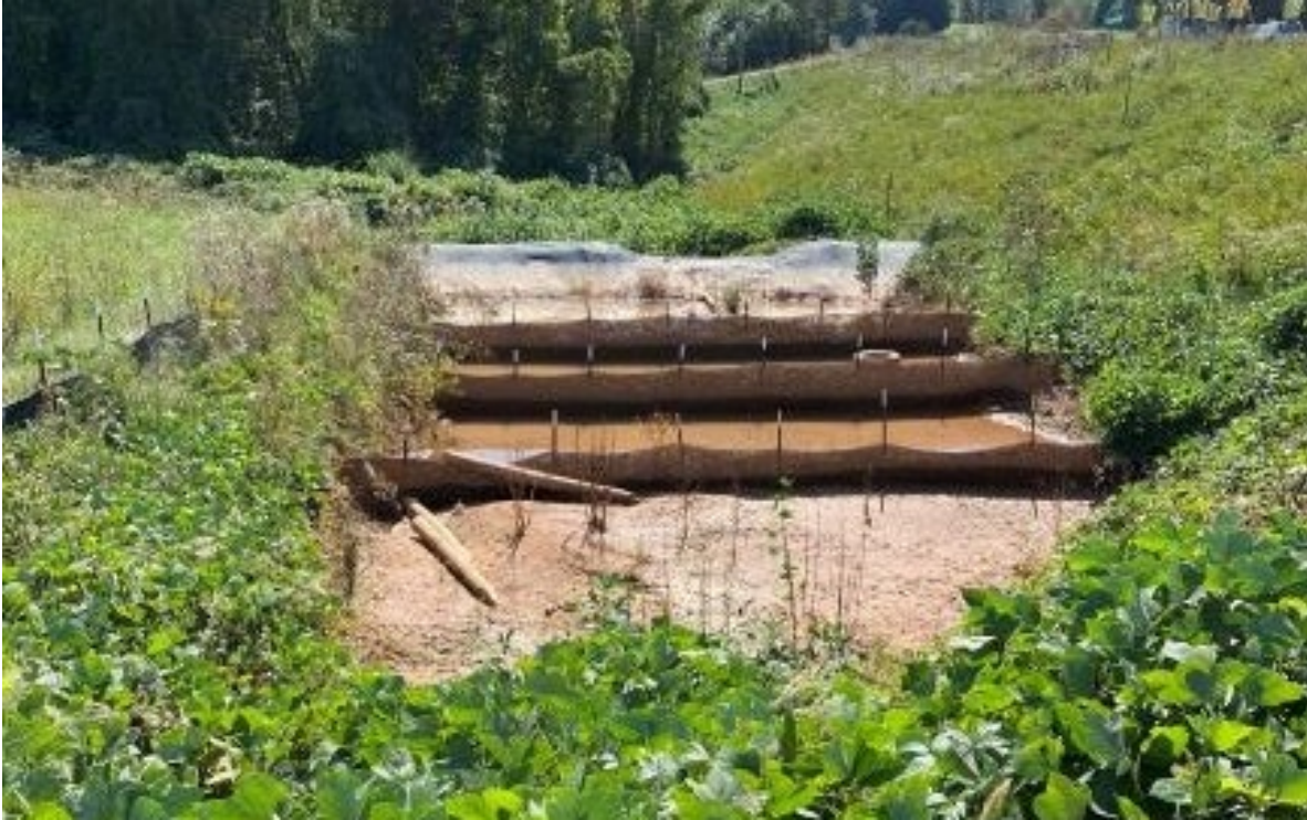
Photo- Wood pole laying across Baffle (10/13/21)
