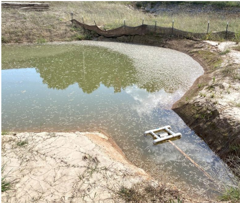
Photo- Basin needing maintenance and skimmer outlet did not daylight (9/29/21)
