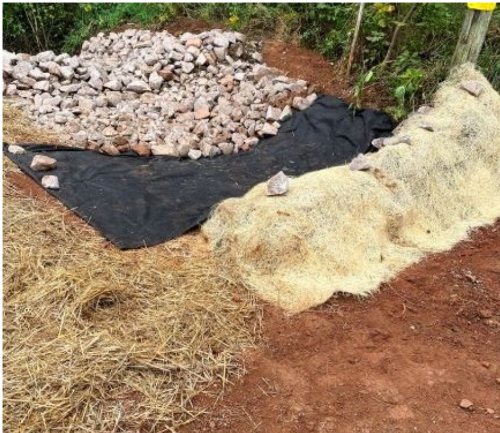
Photo- Bridge #255 over Grant's Creek - Check Dam susceptible to wash around (9/16/2021)
