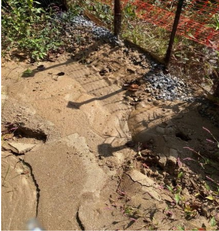
Photo- SSCF needing maintenance (10/14/21)
