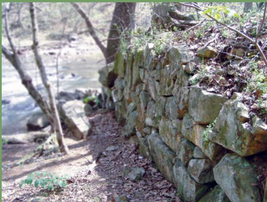
Figure 42 - Ruins of Holden Mill dam constructed of granodiorite blocks.
