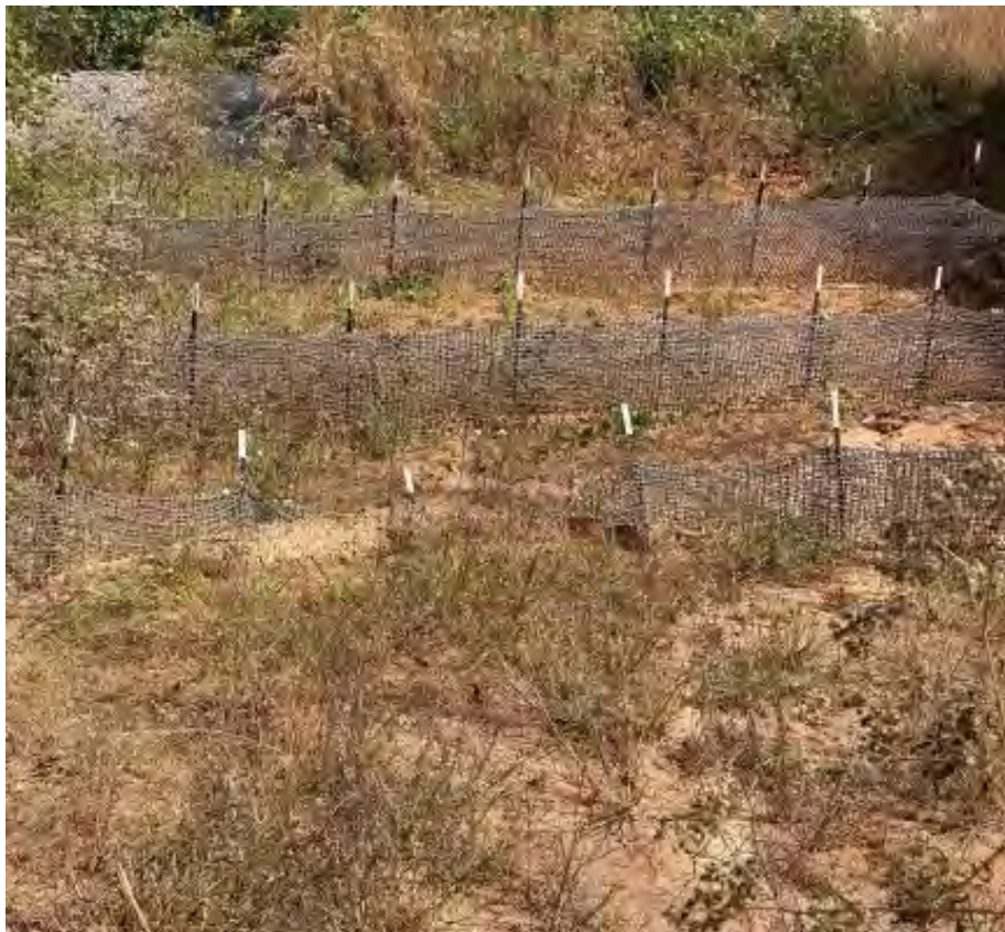
Photo- Section of first baffle knocked down in TRSD-B (10/13/21)
