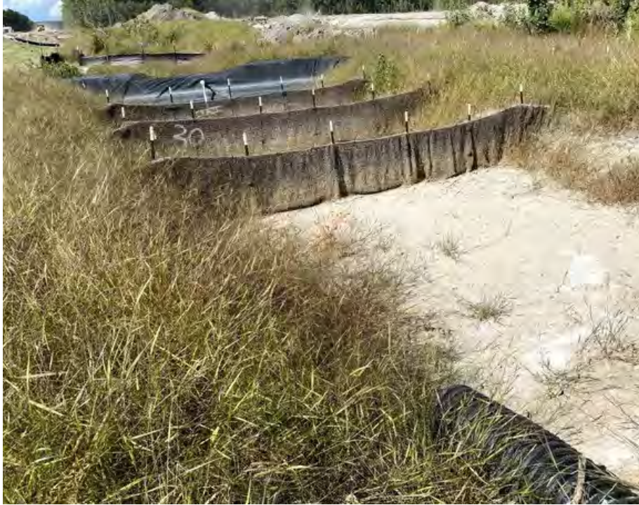
Photo- Skimmer Basin. (10/4/21)
