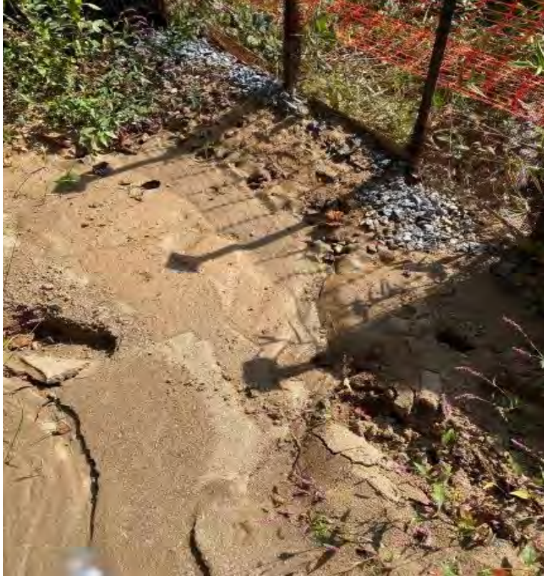
Photo- SSCF needing maintenance (10/14/21)
