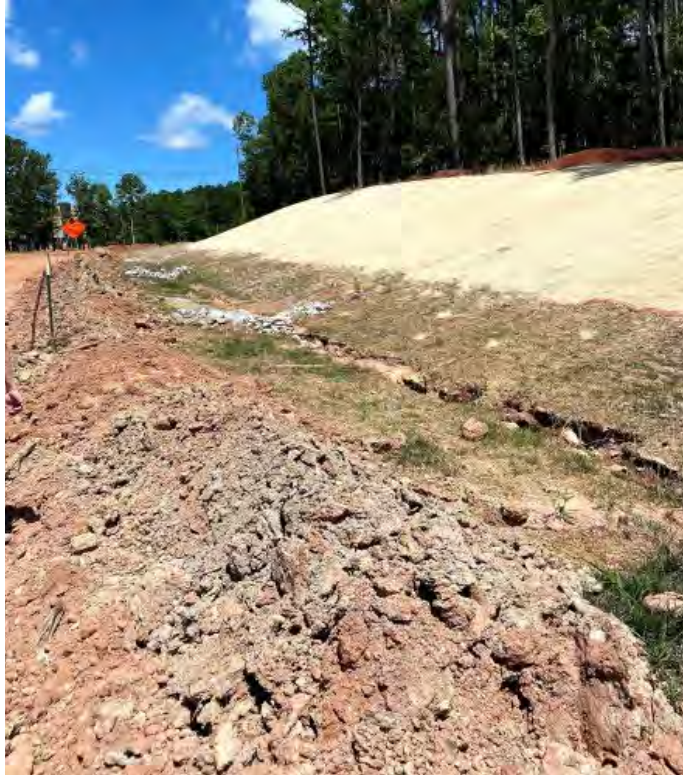
Photo- Ditch bottom beginning to erode. (7/14/2021)
