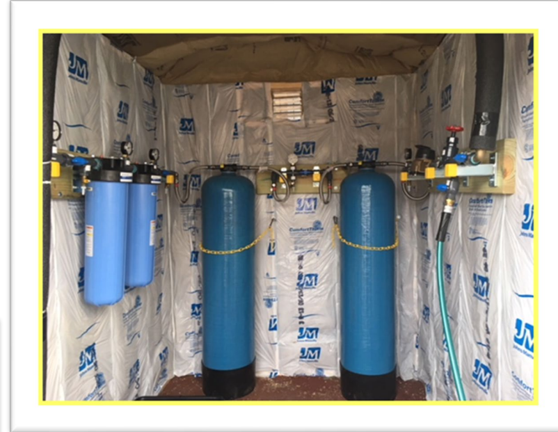
Whole-House Granular Activated Carbon system
