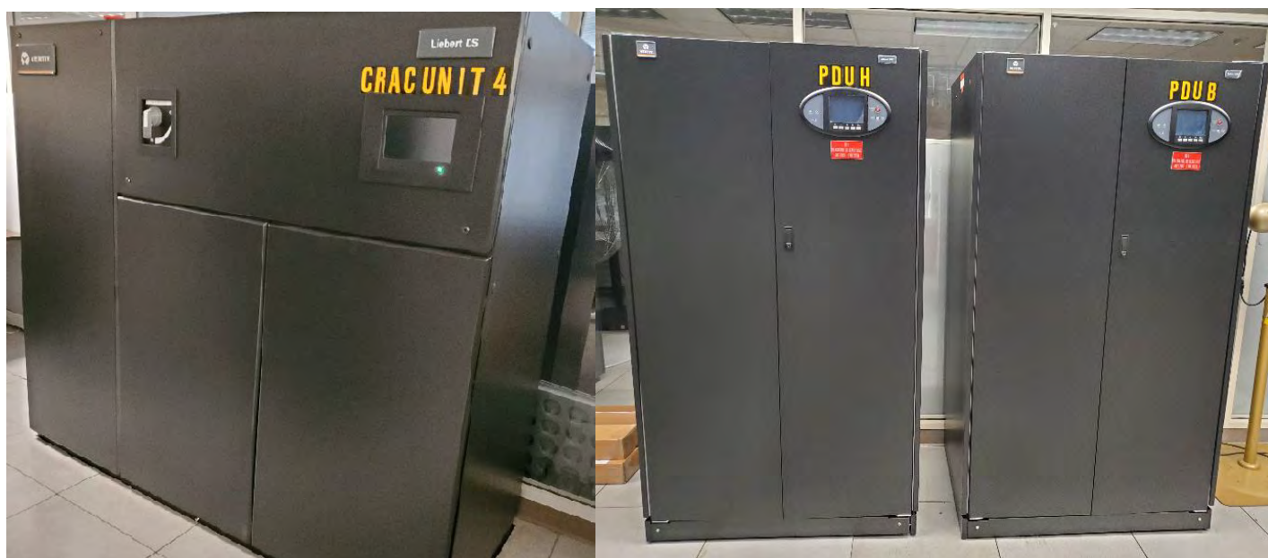
Newly installed equipment inside of our Data Center
