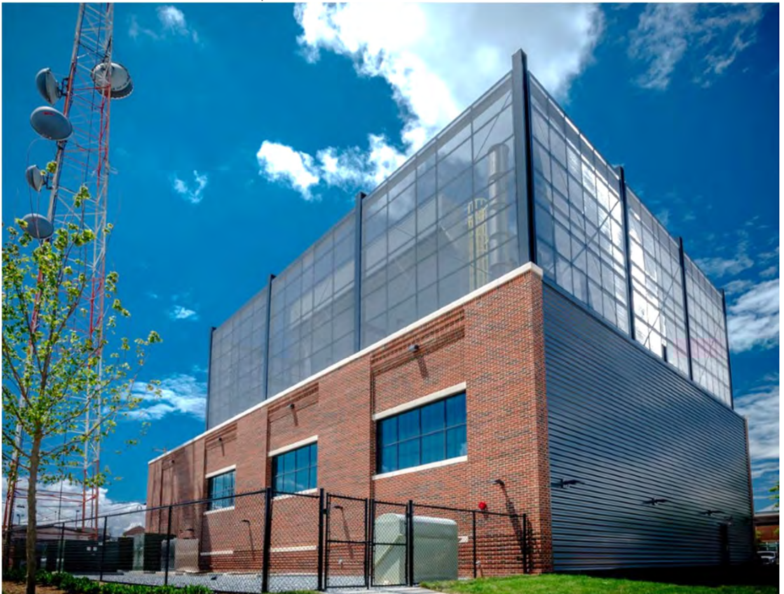
UNC Greensboro South Chiller Plant September 2020
