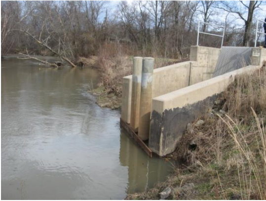
Asheville Water Intake Structure
