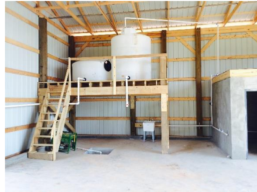
Chemical handling facility- interior
