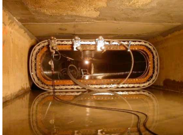
Figure 4-12. Grout-in-Place Spiral-Wound Liner in a Rectangular Cross Section (Courtesy Sekisui SPR Americas, LLC)
