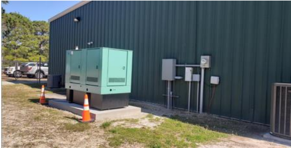
Figure 6.10 – Example of a backup generator elevated to FEMA’s Base Flood of +3 feet of sea level rise inundation.
