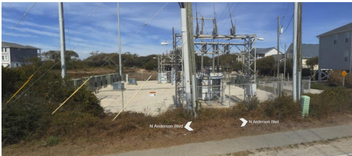
Figure 6.9 – Electrical substation in Topsail Beach near Sidbury Ave. and N. Anderson Blvd. (Bing Maps, 2022)
