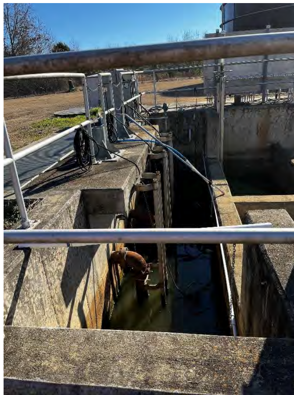
Effluent Pump Station
