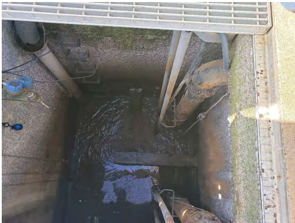
Intake Pumps 1 & 2's Shared Wet Well
