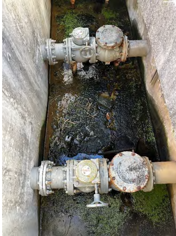
Effluent Pump Check Valves
