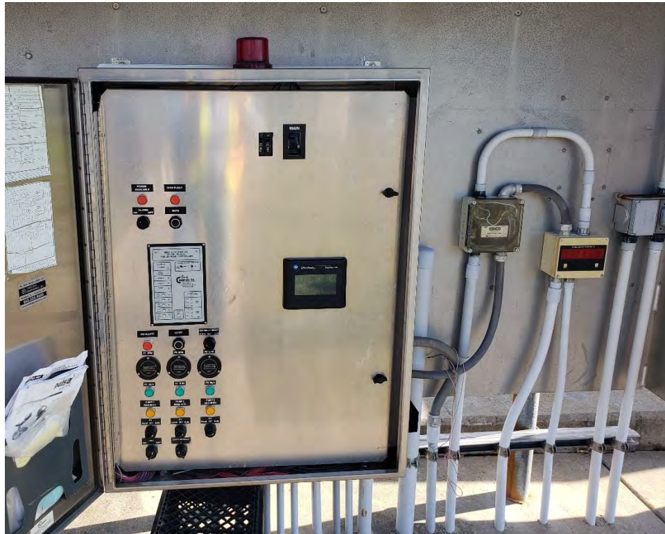
Influent Pump Control Panel
