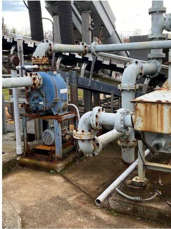
Belt Conveyor, Grit Pump, and Classifier
