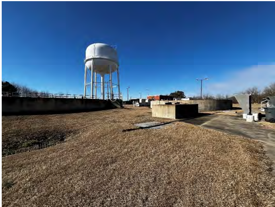
Flow Splitter Box
