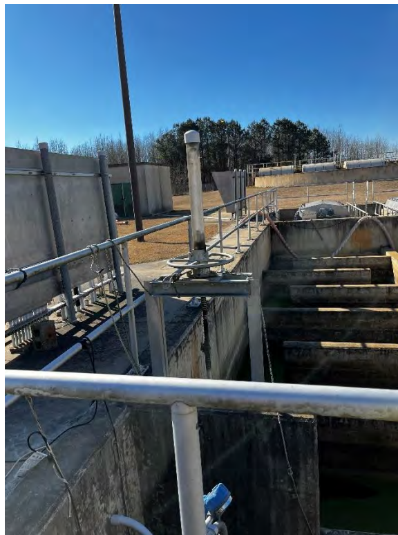
Permanently Closed Slide Gate
