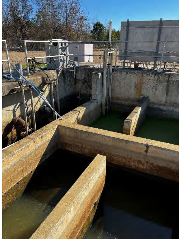
Chlorine Contact Chamber
