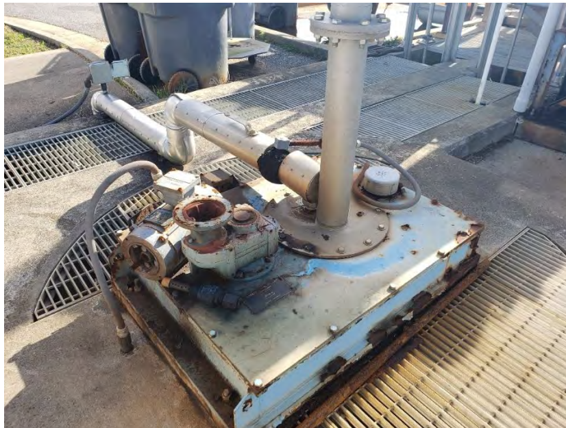
Grit Chamber from Above Access Grate (Side 2)
