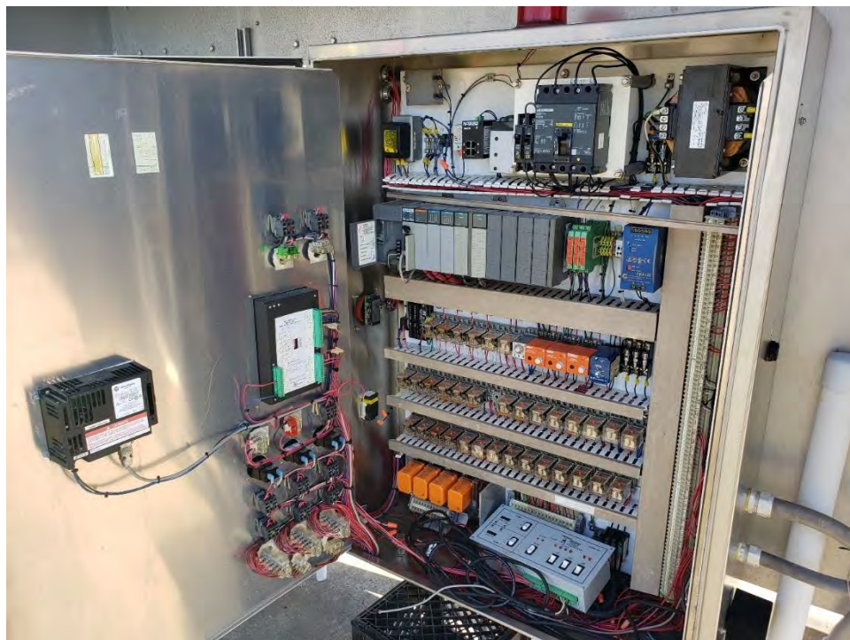
Inside of Influent Control Panel
