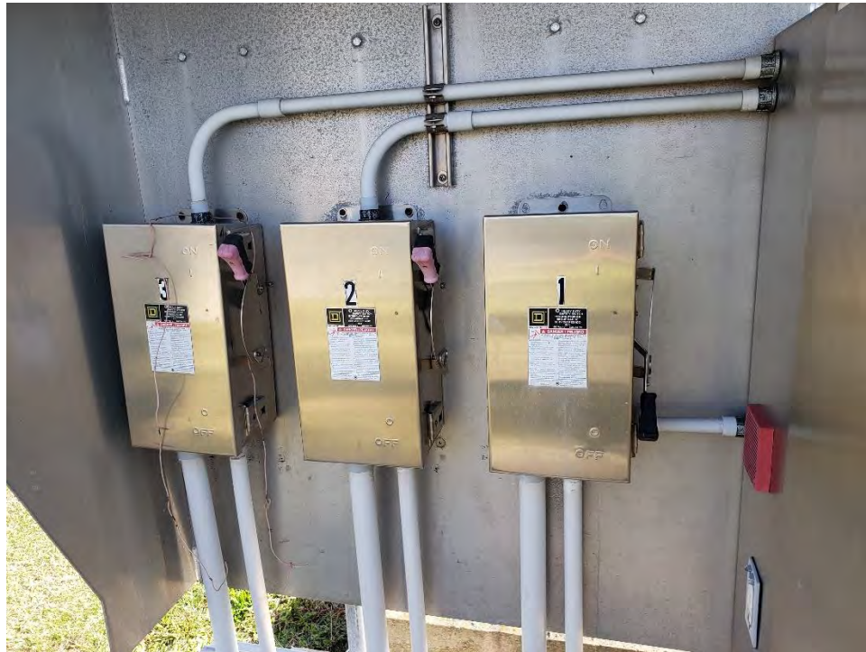
Safety Switches 1, 2, & 3 at Influent Control Panel
