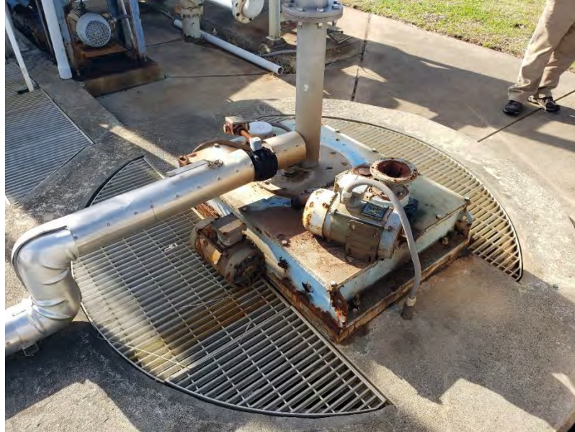
Grit Chamber from Above Access Grate (Side 1)
