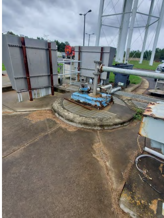
Grit Chamber and Panels
