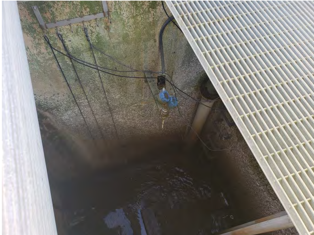
Intake Pump 3's Wet Well
