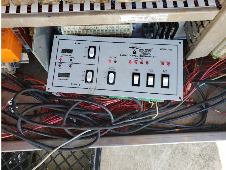
Temporary Dual-Pump Controller for Influent Pump Station Controls
