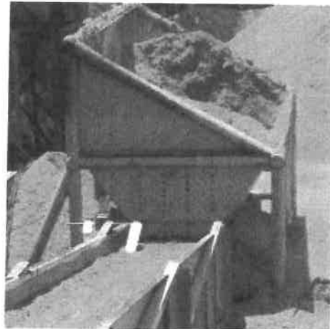
Figure 4-1. Residuals Hopper and Discharge Conveyor
