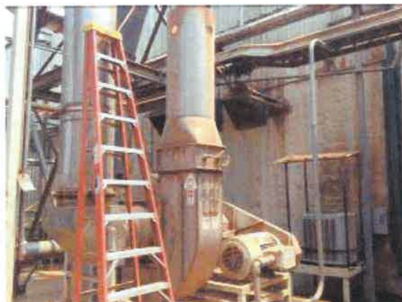
Figure 4-10. Photograph of the Pellet Cooler 2 Stack
