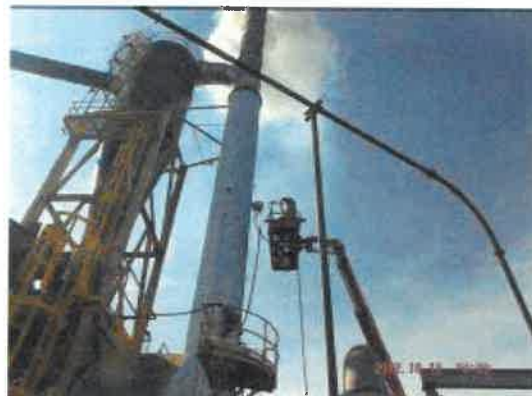
Figure 4-4. Photograph of the Dryer 2 Stack
