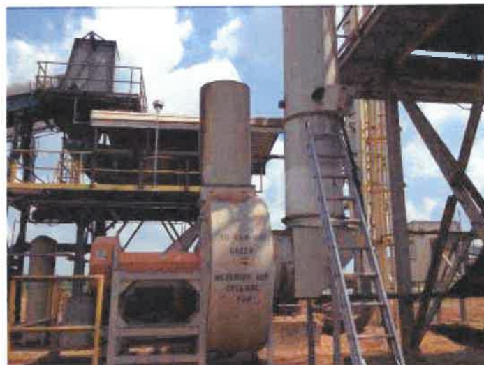
Figure 4-14. Photograph of the Green Hammermill Fan Inlet
