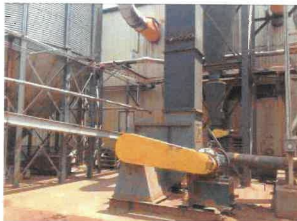
Figure 4-12. Photograph of the Pellet Mill 1 Cooler Stack
