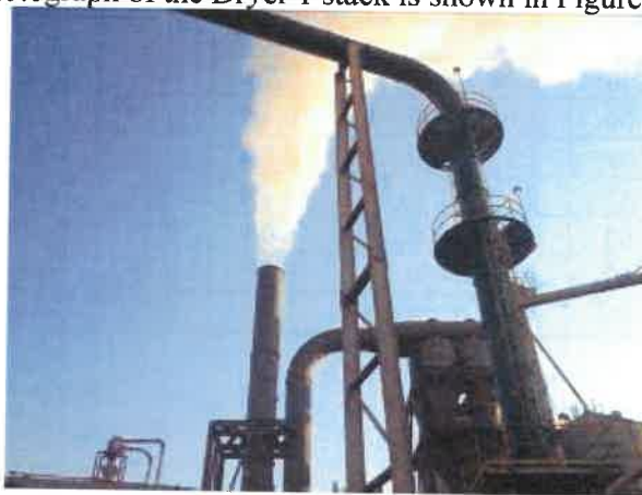
Figure 4-2. Photograph of the Dryer 1 Stack
