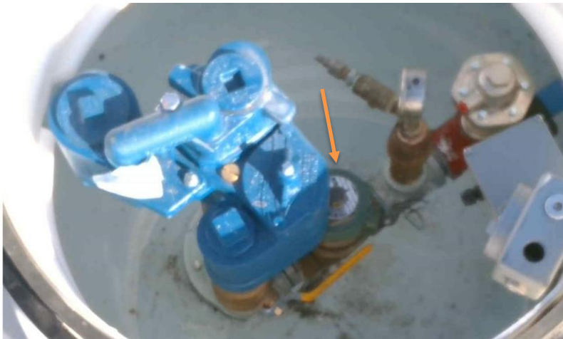
Figure 1: Proper installation of the anti-siphon valve between the STP and Automatic Line Leak Detector
