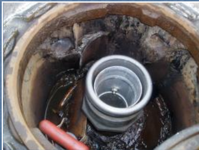
Broken spill bucket
