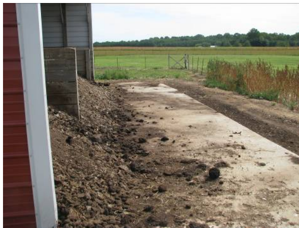
Photo 9. This storage structure may have inadequate capacity for the amount of litter being stored. The area around the storage shed drains to a water of the U.S. and does not have any runoff controls. (Source: EPA Region 3.)
