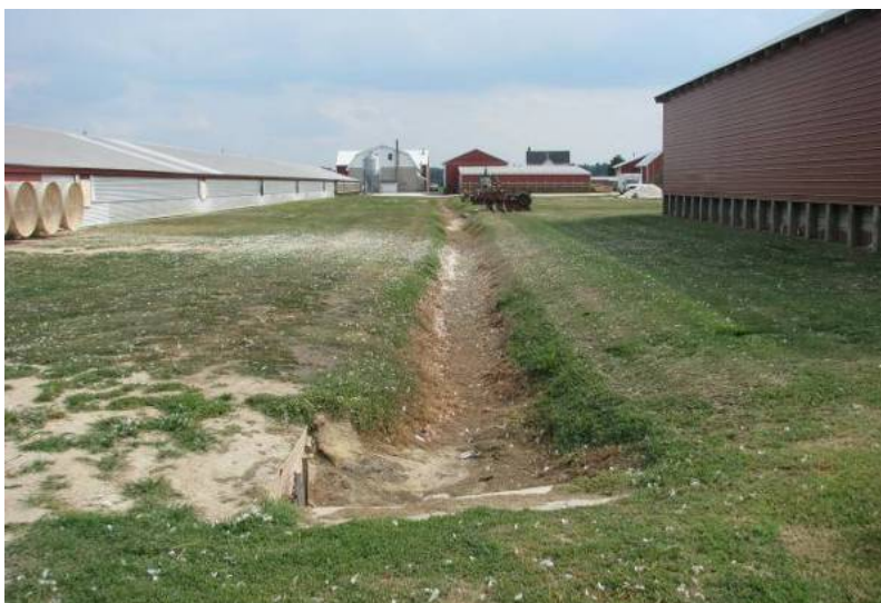
Photo 10. The photo shows a poultry operation that was designed to have precipitation drain away from houses through a conveyance system that discharges to a water of the U.S. If pollutants will be carried by this conveyance system to waters of the U.S., the facility is proposing to discharge. (Source: EPA Region 3.)
