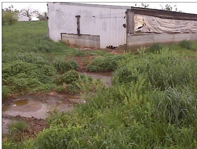
Photo 8. An in-house pit in this swine barn is designed to have manure transported from the pit to an earthen storage structure through a pipe. Due to a pipe break, manure is leaking and flowing downhill from the barn. (Source: EPA Region 5.)
