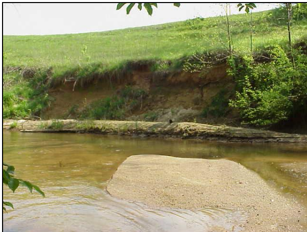
Figure 7. Bank erosion and lack of riparian zone (North Little Hunting Creek, SR 1829, Iredell County).
