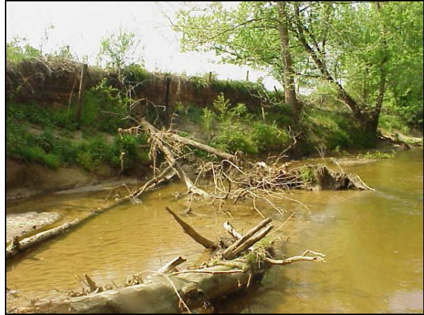
Bank erosion in North Little Hunting Creek, SR 1829, Iredell County.
