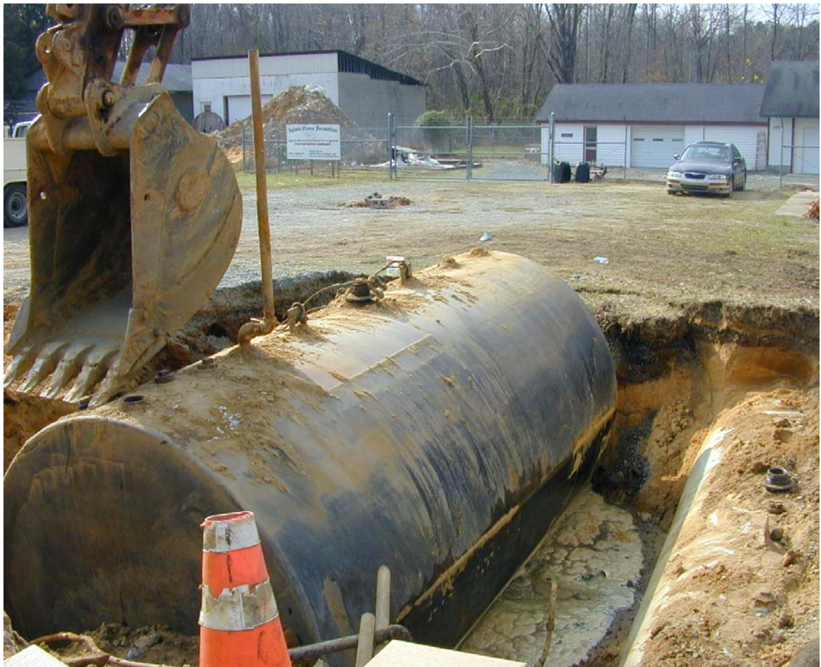
UST Release Incident-Kerosene Free Product in Basin
