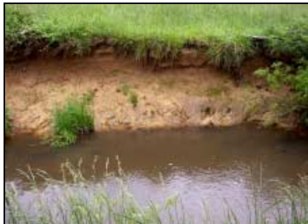
Figure 4. Eroding vertical banks, Rocky River, SR 1300, Chatham County.
