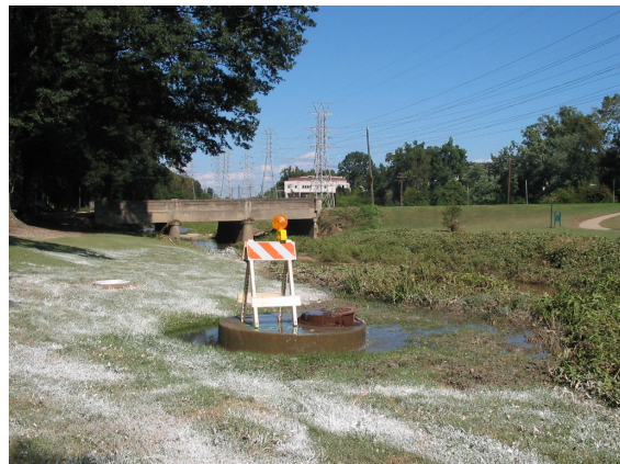
Sewer system overflow draining into North Buffalo Creek within subwatershed 4. The City of Greensboro maintains a database of SSOs as part of a program to minimize the occurrence of uncontrolled discharges from the sanitary sewer collection system.
