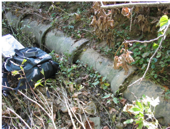
Aging sanitary sewer lines, especially those constructed with short sections (2') of clay pipe as shown above, have the potential to be significant sources of bacterial contamination due to leaks at the joints. Mapping the major components of the sanitary sewer collection system will be an important foundation to future implementation strategies.
