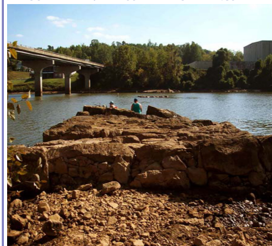
FIGURE 4-12: EXPOSED BRIDGE PILINGS
