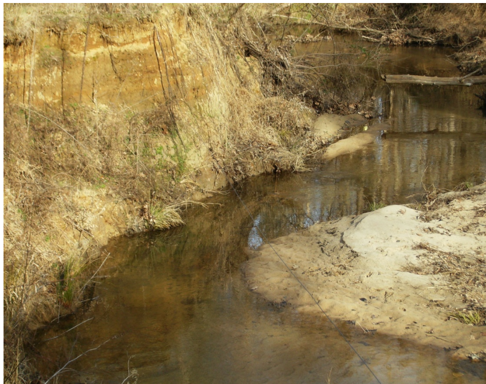
Example of bank erosion located at the Rattlesnake creek in Caswell County. This Stream is in need of restoration work to stabilize the banks from excessive erosion.
