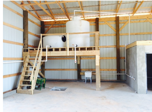
Chemical handling facility- interior
