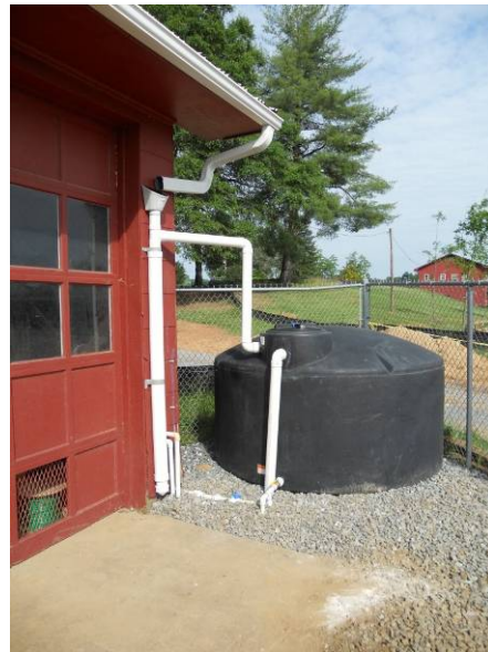
An above-ground cistern located at the City of Morganton Parks and Recreation maintenance building catches runoff from the roof. The water is used to clean equipment.
