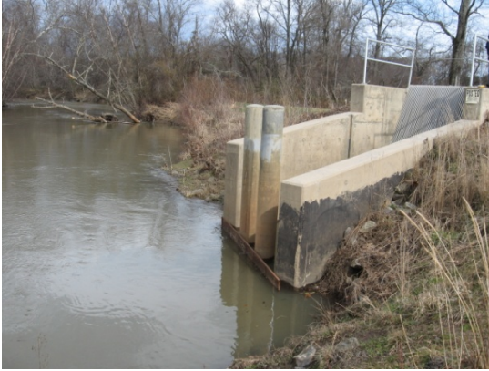
Asheville Water Intake Structure
