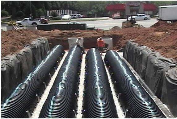
Filtration chambers are installed during construction of the Bojangles parking lot in Morganton (outside the Hunting Creek Watershed). The chambers will capture stormwater and filter it through a sand and stone medium before releasing it to a nearby stream.
