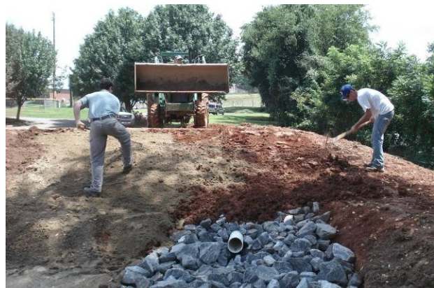
...and enters the bio-retention area through an underground pipe.
