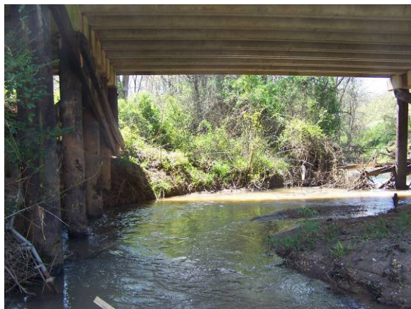
Bridge crossing not aligned with flow of stream causing stream bank erosion.
