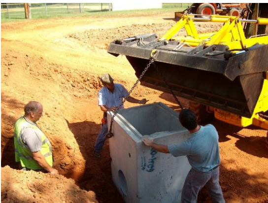
A stand pipe is placed within the bio-retention area to direct overflowing water back into the storm system in the event of large rainfall.
