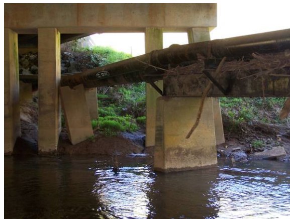
Pipe utility crossing Hunting Creek under US-70 bridge. Note dislodged footer causing sag in pipe at joint.
