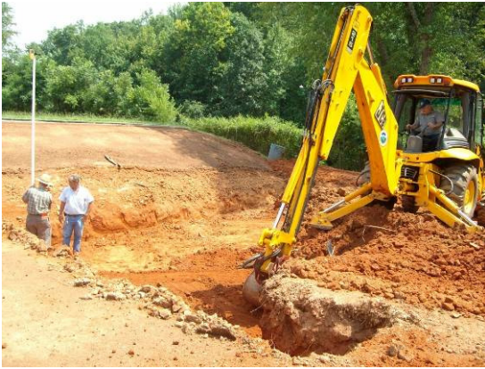
A depression is being dug for the installation of a bio-retention area at Gene Turner Park in Morganton outside the Hunting Creek Watershed.
