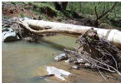
Pipe utility crossing Hunting Creek above stream with debris pile behind pipe. Also note erosion along stream bank
