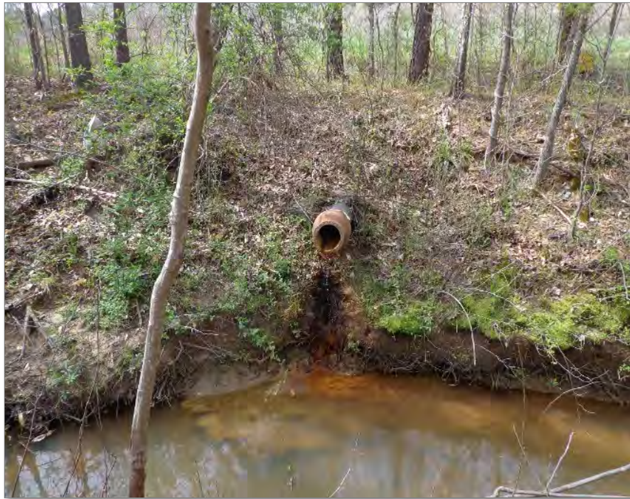
Photo 4. Example of Pipe Discharging to Stream from Unknown Source
