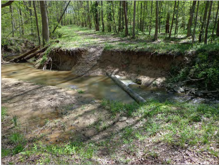
Photo 6. Exposed sanitary sewer line due to bed and bank erosion.
