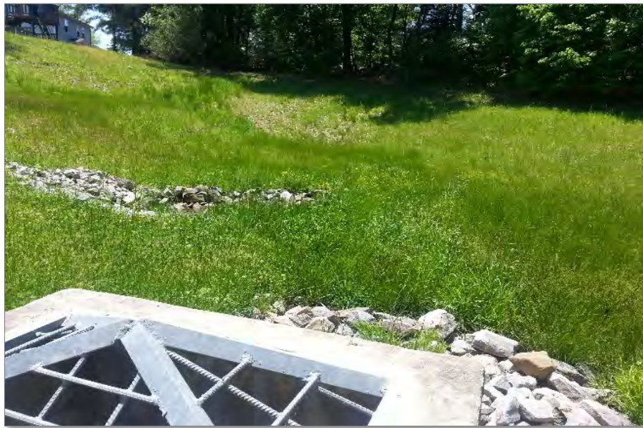
Photo 17. SCM 00161 – Example of a potential volume and structural retrofit combination that would increase SCM volume and treatment time
