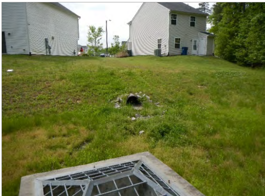
Photo 19. SCM 00354 – Example of a short circuited flow path with inlet directly across from outlet
