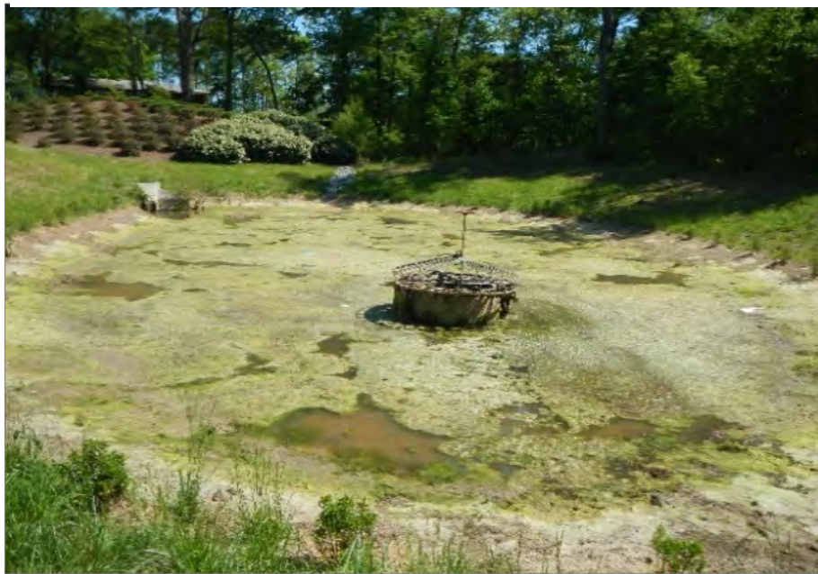
Photo 12. SCM 00390 – Clogged riser orifice leading to heavy algae growth and limited capacity
