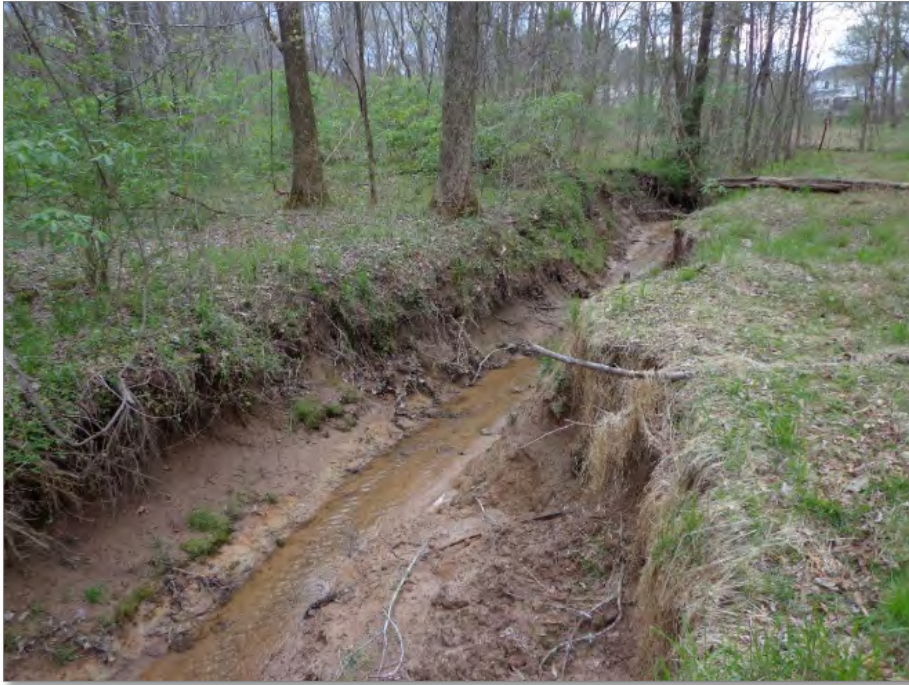
Photo 1. Example of Poor Overall Stream Condition
