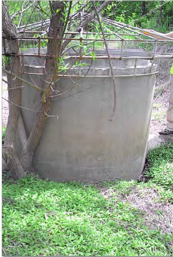
Photo 13. SCM 00420 – Woody vegetation growing in footprint and endangering riser structure
