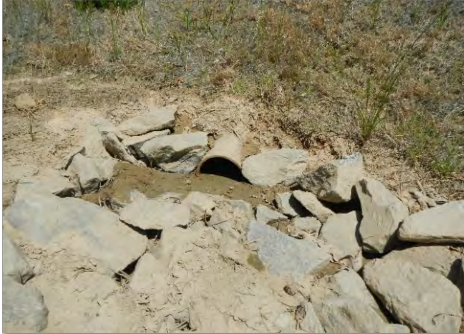
Photo 11. SCM 00777 – Inlet pipe to level spreader clogged with 2" sediment
