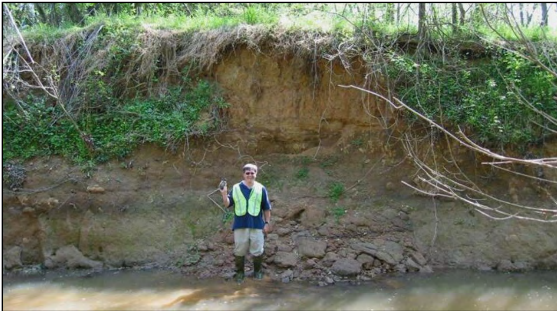
Figure 10: Significant Channel Incision (Scour) on McDowell Creek.
