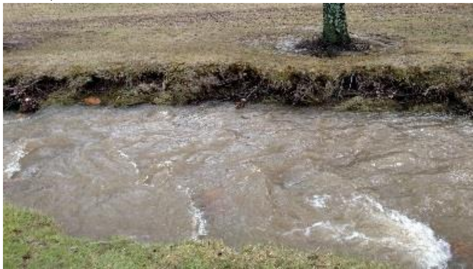
Figure 8. The picture above, taken at Foster Tyson Park, is an example of a destabilized bank.
